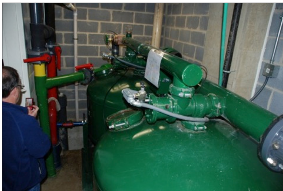
Figure 4.6. The clogged sand filters in the pump room of the WIMSA CWF. Photo taken on October 24, 2014.
