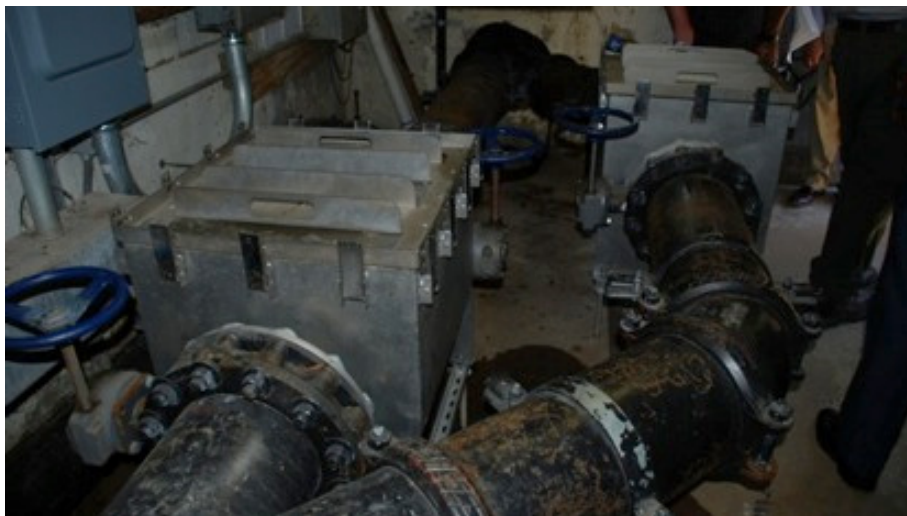
Figure 3.5. The screen filters in the pump room at Meridian Hill Park.
