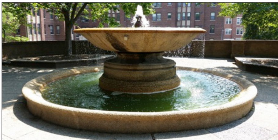
Figure 3.28. Blackish staining underneath the top fountain basin. Photo taken July 1, 2014.
