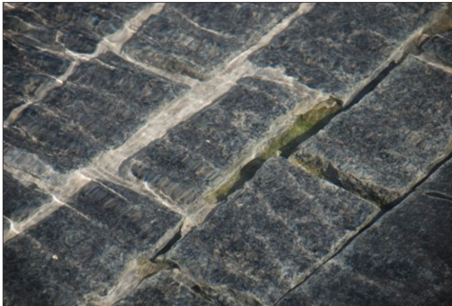
Figure 4.13. Algae are difficult to clean when it lies in the space between cobblestones. Photo taken October 24, 2014.
