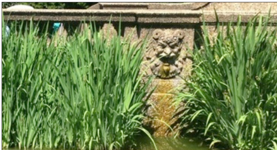
Figure 3.27. Greenish staining, likely from biofilms and algal growth on the walls of the CWF. Photo taken June 6, 2014.
