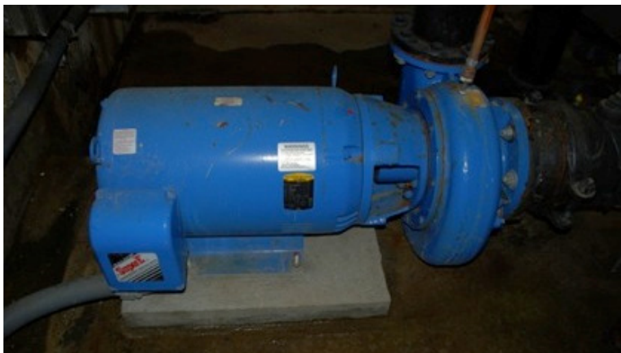
Figure 3.3. The 60-HP pump at Meridian Hill Park.
