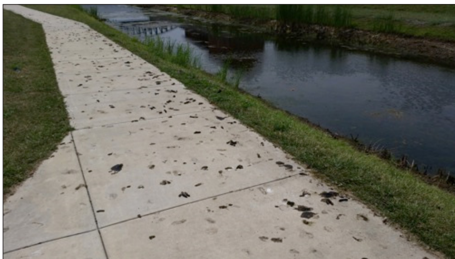
Figure 6.29. Bird droppings along the walkways along the CHOH Canal basin. Photo taken July 7, 2014.
