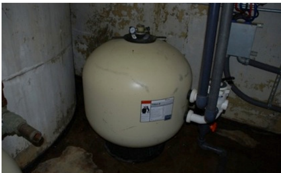
Figure 3.4. One of the sand filters in the pump room at Meridian Hill Park.
