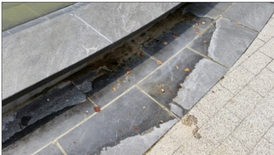
Figure 4.5. Leakage along the sides of the reflecting pool. Photo taken August 6, 2014.
