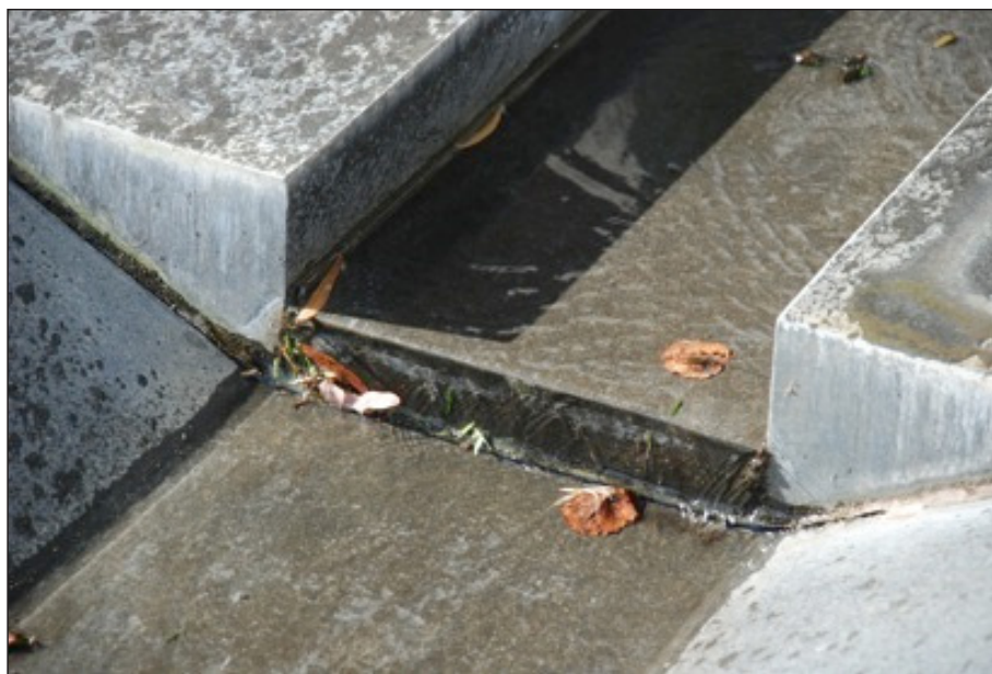
Figure 4.12. Plant debris collecting in the narrow channel on October 24, 2014.
