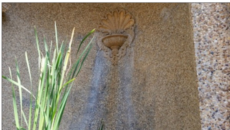
Figure 3.26. This photo shows the stains on the walls of the CWF. Photo taken June 6, 2014.
