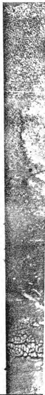
Visitor's Center - West Ele. Interior side of Parapet. Extensive step cracking is visible.
