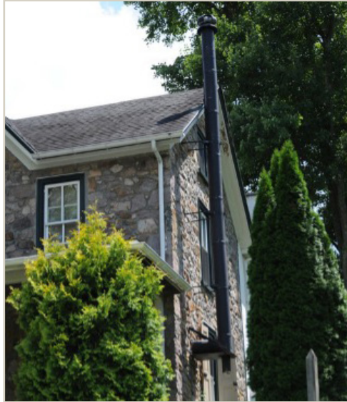
External metal flues are inappropriate appendages to historic resources and should be avoided as they detract from the historic character of the resource.
