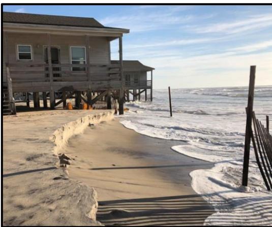
An extreme high tide in December 2019 washes under the Long Point Cabins and cuts a scarp in the sand. These flood events will become more common as sea levels continue to rise [NPS].
