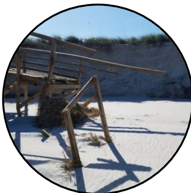
A boardwalk ramp at Fort Matanzas washed out by Hurricane Matthew in 2016 [NPS].
