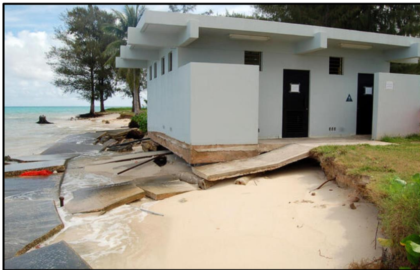
The damaged public bathrooms at their original location [NPS]
