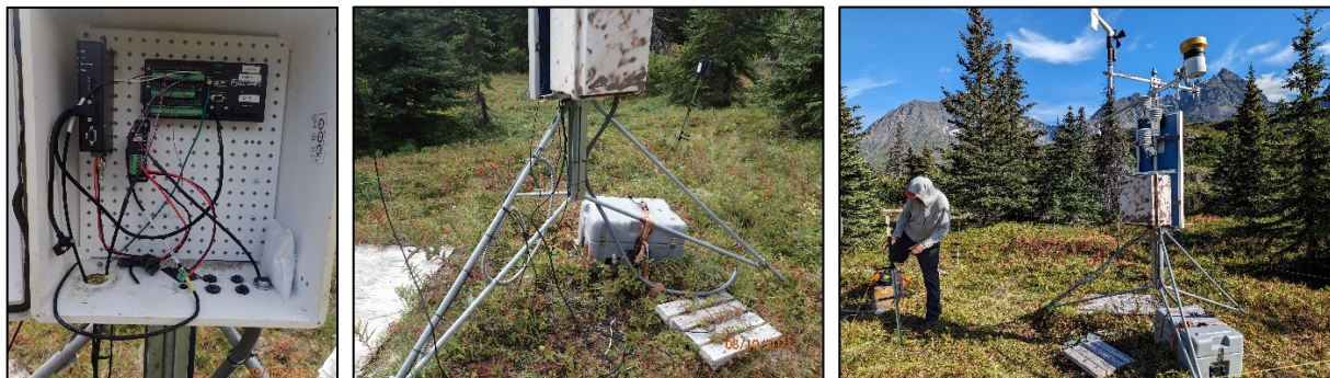
Figure 11. Tebay climate station, August 19, 2023. Site had been damaged (left and center). Station after site maintenance was completed (right).
