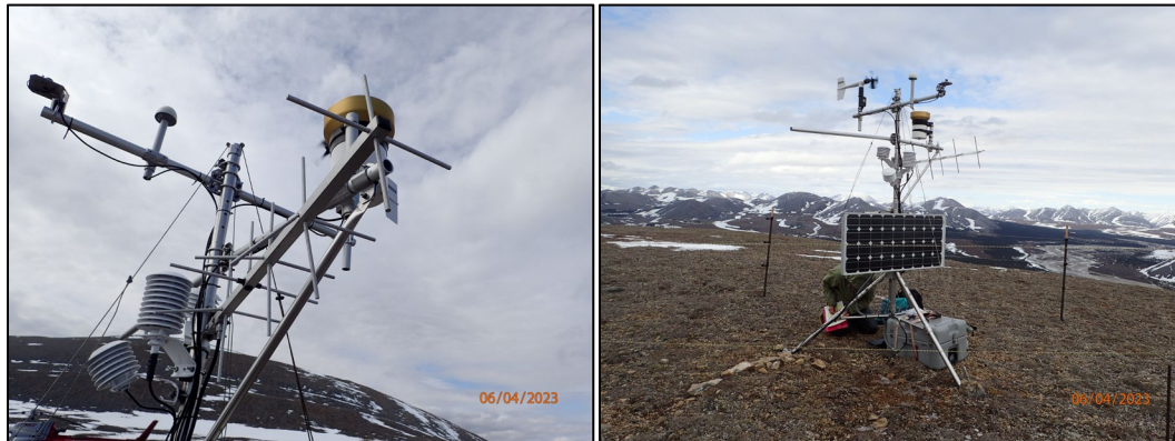
Figure 6. Asik climate station June 4, 2023. The Yagi antenna was damaged and out of alignment (left). The station at end of site visit (right).
