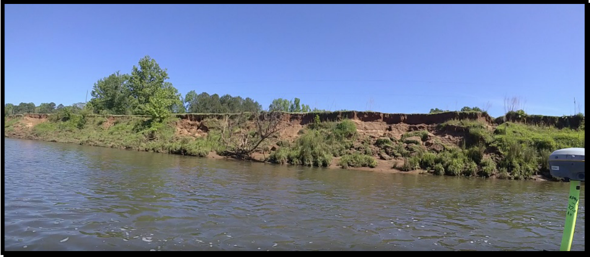
Figure 23: An example of a degraded streambank observed upstream of HOBE on the Tallapoosa River.
