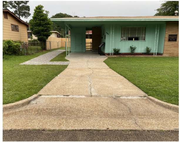
FIGURE 3–24. The concrete driveway is visibly worn and has significant cracking (source: DHM Design, 2023).
