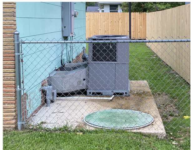
FIGURE 3–40. HVAC utilities at the Medgar and Myrlie Evers House NHL (source: DHM Design, 2023).
