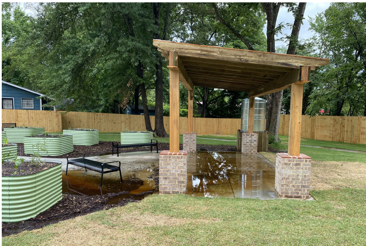
FIGURE 3–14. At the Missouri Street Lots, drainage issues at the shade structure occur after a large storm event (source: DHM Design, 2023).
