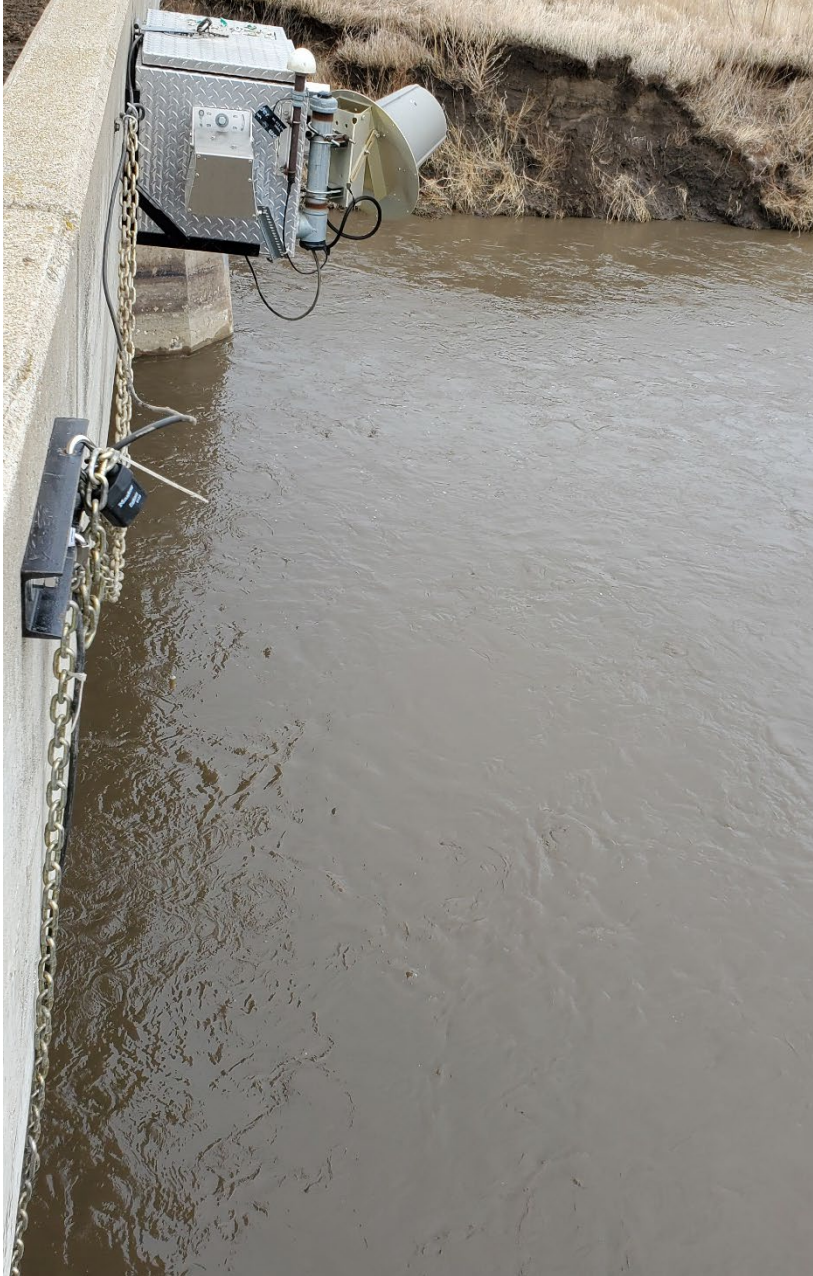
Figure 3. The radar head for the gage is attached to the bridge at station 06478522, Bow Creek.
