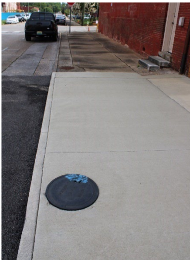
FIGURE 3-20. Manhole covering the water meter that serves the Bus Depot, looking east, 2021. Laura Knott.
