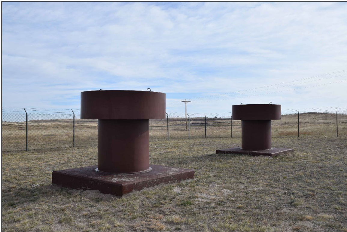
Photograph 27. Air intake duct (left) and air exhaust duct (right). View east-northeast.
