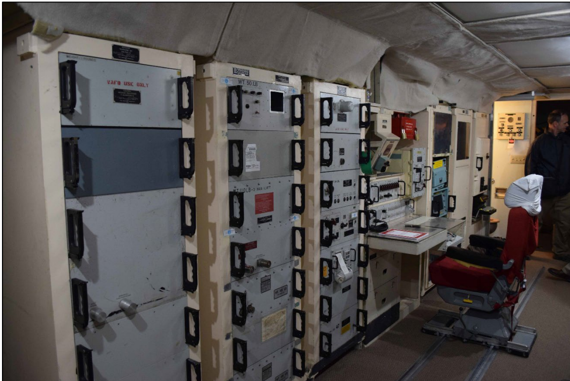
Photograph 9. The west wall of the LCC holds computer racks (left), the DMCCC's console with the red, double-padlocked, launch key safe above, and a latrine in an alcove at the end. View north-northwest.
