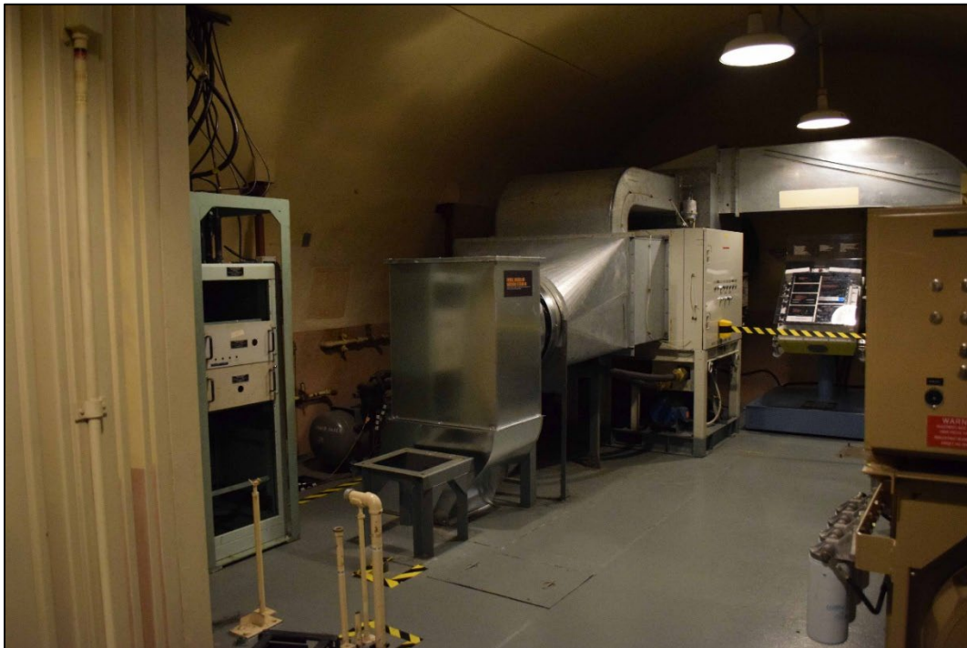
Photograph 12. The west wall of the LCEB holds the brine chiller (far right) with chemical, biological, and radiological filters and a fan unit to the right. An interpretive display stands at the north end. A generator is located on the east wall (right). View northwest.
