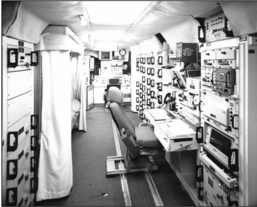
Figure 15. The underground launch control capsule is pictured here, with the missile commander's console at the far end and the deputy missile commander's console to the right in this 1999 photograph. Courtesy of Historic American Engineering Record draft documentation, Photograph HAER WY-89, 1999.
