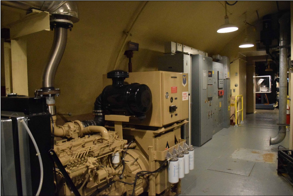
Photograph 13. The east wall of the LCEB contains a diesel electric generator (left) and an automatic switching unit to the right. View south.
