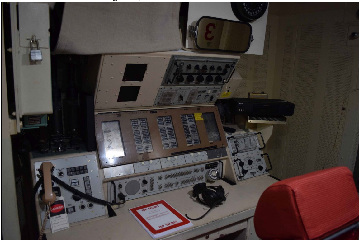
Photograph 8. The commander's console is at the south end of the LCC. Note the mirror and 24-hour-clock (above right). View southwest.
