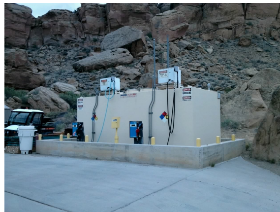
2018_CHCU_72077_Diesel Fueling Tank_Front.jpg
