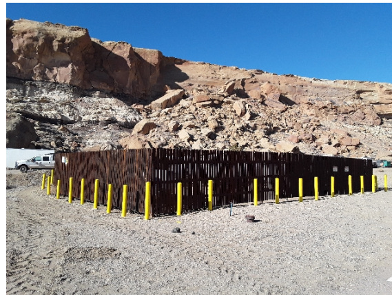
2021_CHCU_92309_Ast. Propane Tank Group_Front.jpg
