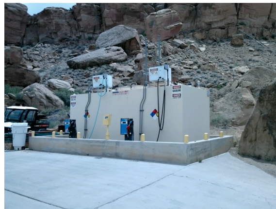
2018_CHCU_72073_Gas Fueling Tank_Front.jpg
