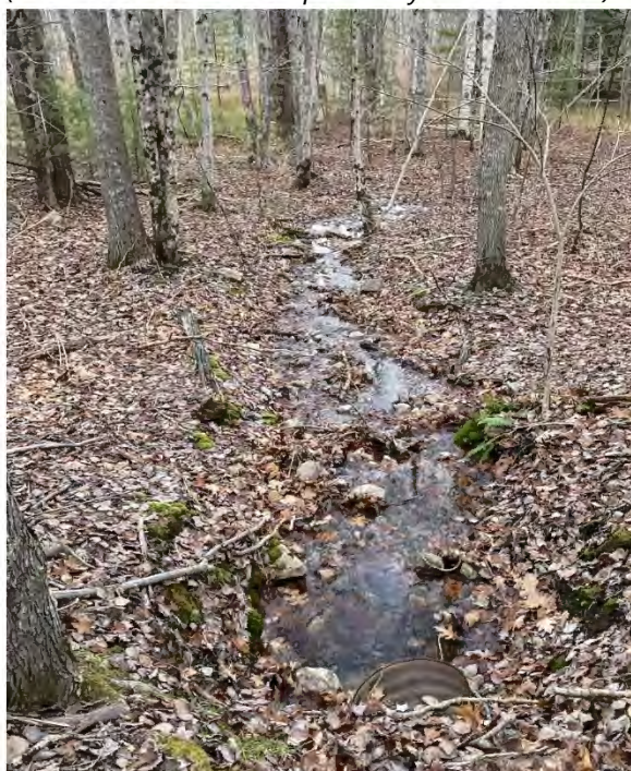
Photo 10: Culvert under Hemlock Path (Hemlock-2). Scour and sediment deposits observed at culvert outlet.
