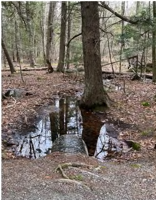
Photo 13: Southern culvert under Hemlock Path (Hemlock-6). Downstream erosion observed at culvert, with a significant scour hole at the outlet.
