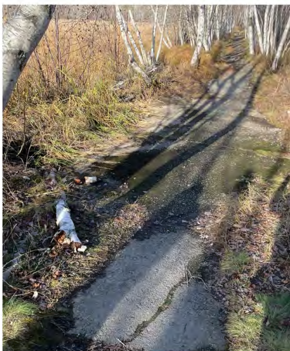
Photo 15: Culvert under Hemlock Path (Hemlock-7). The concrete low-water crossing only conveys flow under flood conditions, and presents a barrier to aquatic organism passage and habitat connectivity.
