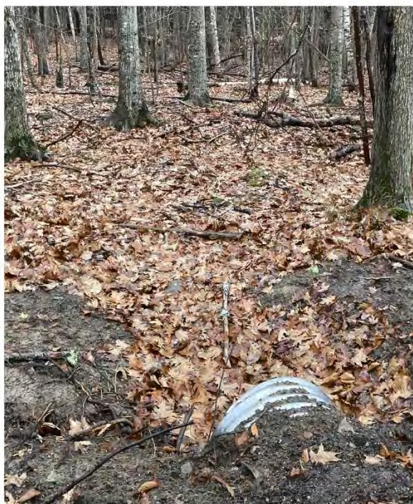
Photo 8: Newly constructed culvert under Sweet Water Circle (Sieur de Monts-1). There is no established drainage path to the culvert inlet. (Note: has since been replaced by dual 18" CMP)
