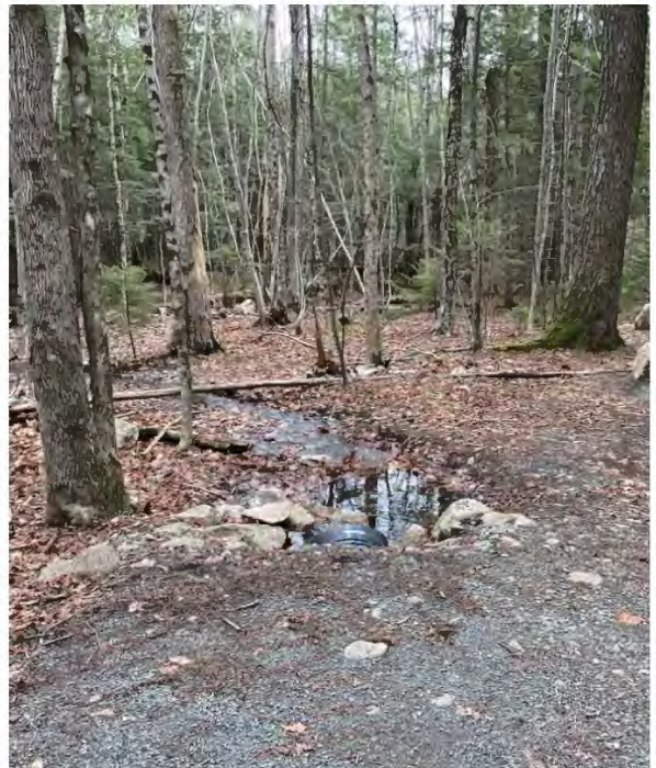
Photo 14: Northern culvert under Hemlock Path (Hemlock-6). Downstream erosion observed at culvert outlet.
