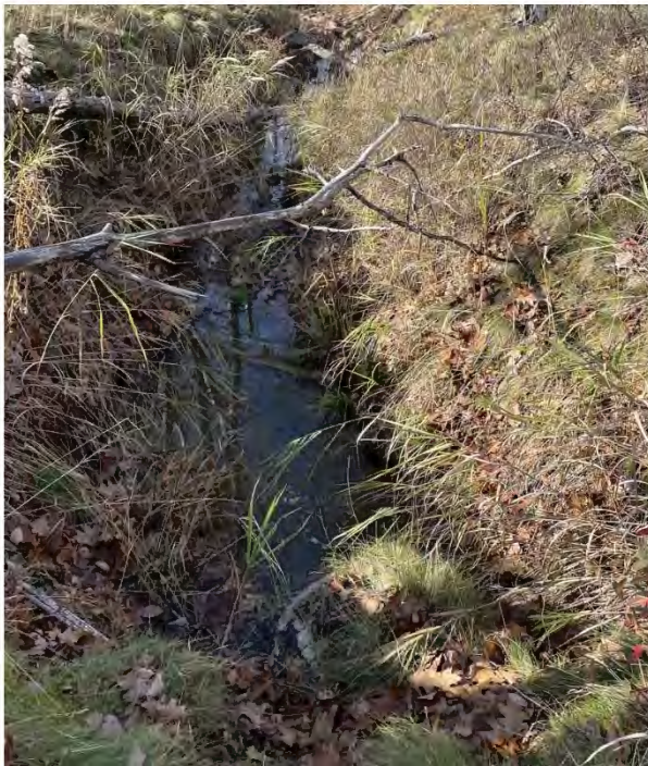
Photo 5: Culvert under Park Loop Road (Park Loop Rd-8). Channel erosion observed downstream due to concentrated flow from culvert.
