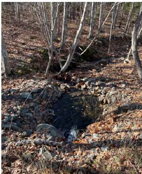
Photo 7: Outlet of culvert under Rt 3 (Route 3-2). Scour pool and major channel erosion observed downstream due to concentrated flow from culvert.
