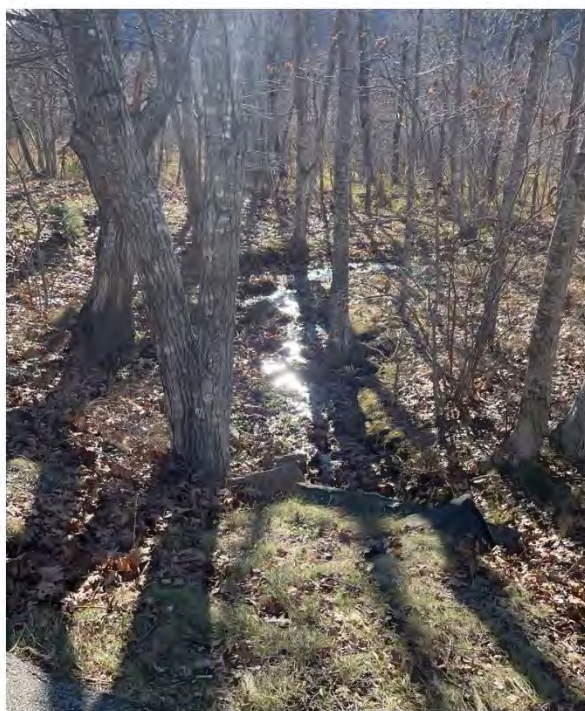
Photo 2: Culvert under Park Loop Road (Park Loop Rd-2). Outlet headwall is collapsing, and channel erosion observed downstream of culvert outlet.
