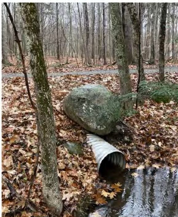
Photo 9: Culvert under service road near Sweet Water Circle. This culvert conveys runoff to an undersized closed drainage system below the visitor center, causing localized flooding.
