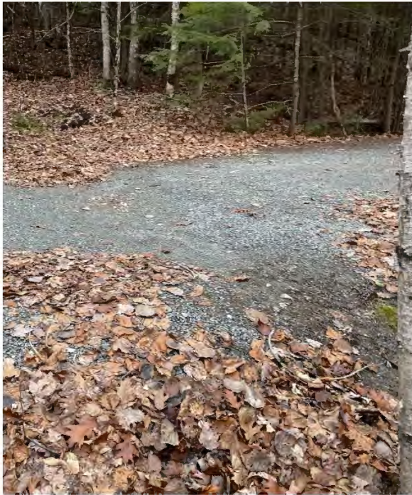
Photo 11: Overland flow over Hemlock Path (Hemlock-3). Flow path observed the path surface, causing areas of erosion.
