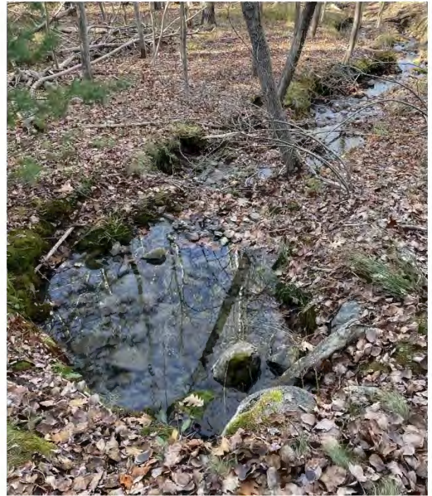
Photo 6: Culvert crossing diagonally under Park Loop Road at Route 3 (Route 3-1). Channel erosion observed downstream due to concentrated flow from culvert.
