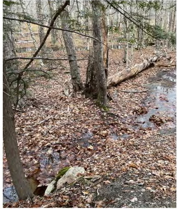
Photo 12: Culvert under Hemlock Path (Hemlock-4). Channel erosion observed downstream of culvert outlet.
