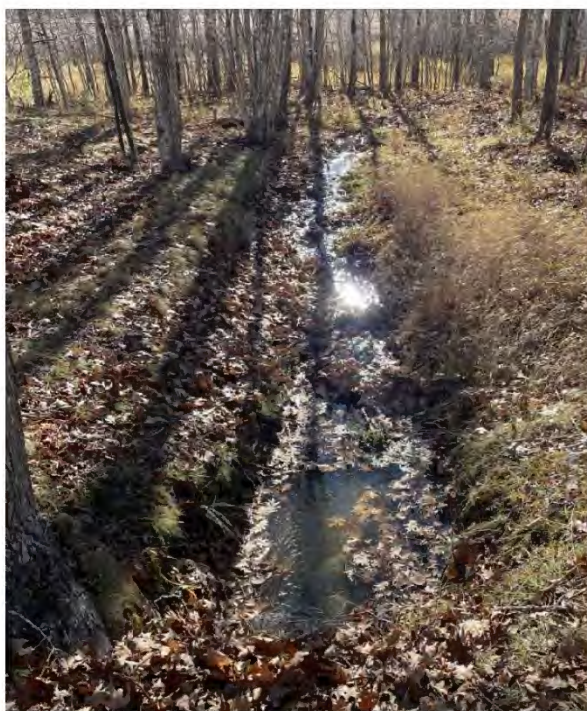
Photo 1: Culvert under Park Loop Road (Park Loop Rd-1). Channel erosion observed downstream of culvert outlet.
