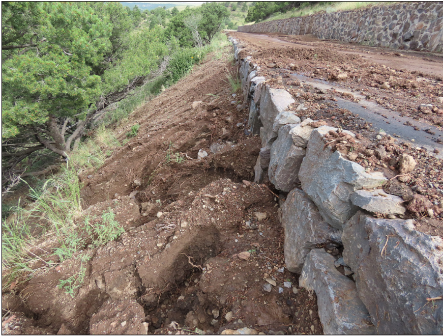
Erosion on the cinder cone at Capulin Volcano NM in 2019. Both vegetation on the cone and Volcano Road, an important part of the monument's cultural landscape, are impacted by erosion from rainfall events like this one in August 2019. Increased amounts of precipitation or intensity of rainfall events associated with a future, warmer climate (e.g., Myhre et al. 2019) could lead to future erosion events like this one. NPS Photo.
