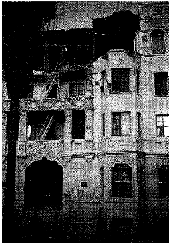
Red tags are intended only to indicate that a building is unsafe to occupy. Many times, however, they are misinterpreted as being a recommendation for demolition.
