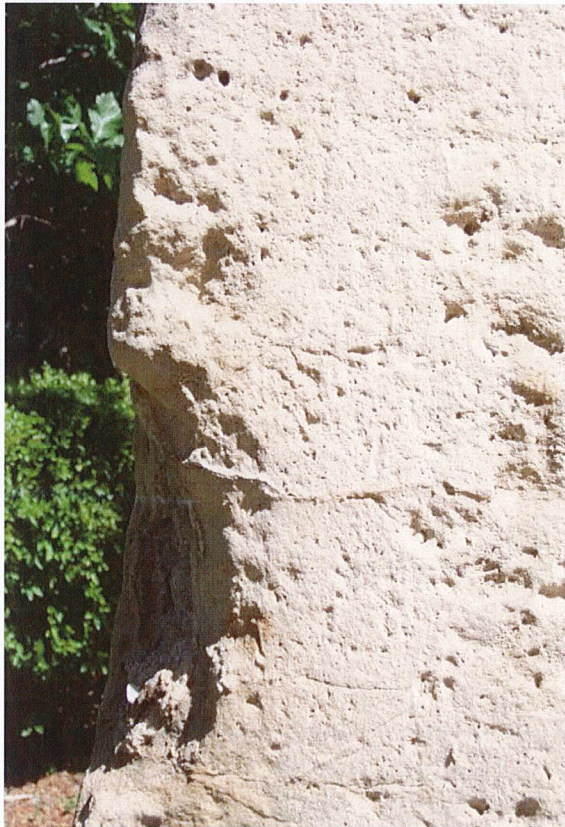
Figure 9. Missing chunk from the monument. June 2017.
