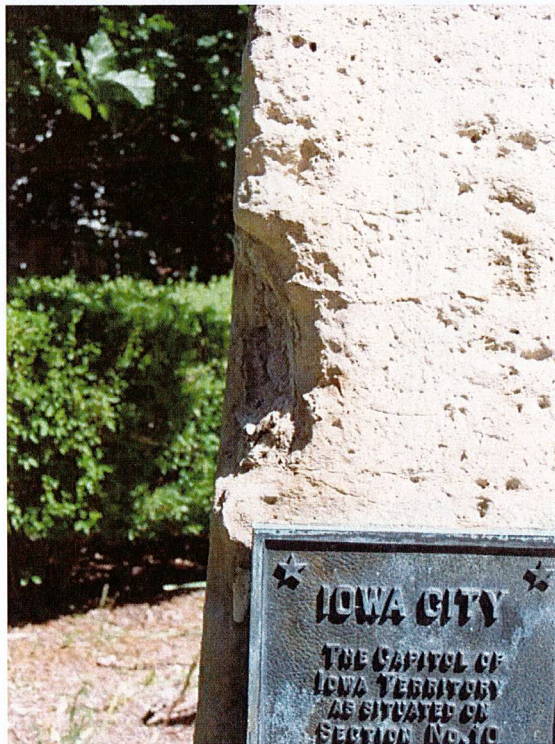
Figure 15. Missing chunk from the monument. June 2017.
