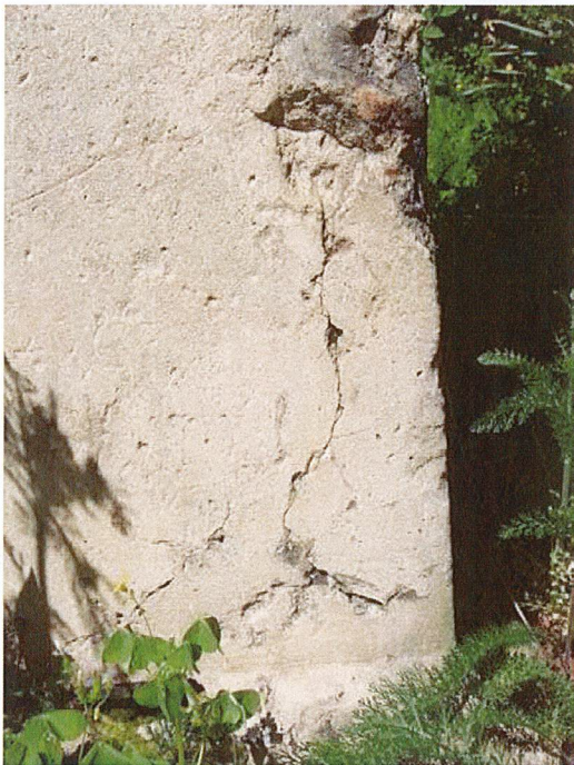
Figure 12. Cracking located at the lower portion of the monument. June 2017.
