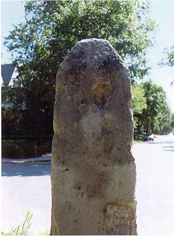
Figure 14. Cracks and holes in the limestone. June 2017.
