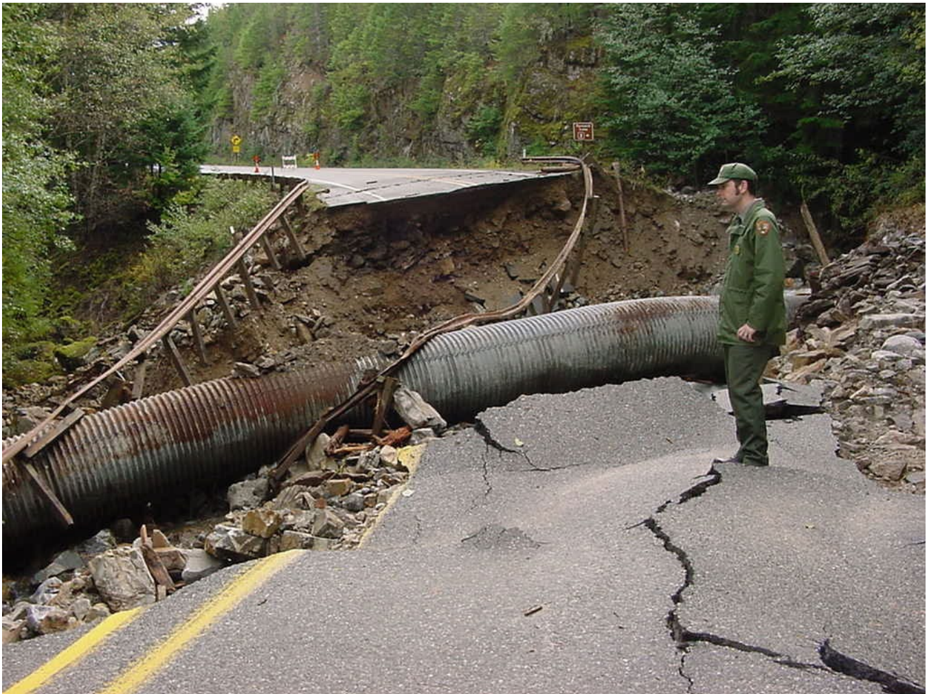
Figure 8. Photograph of roadway and culvert damage following a landslide in 2003. The landslide event occurred near Pyramid Creek in ROLA and has wiped out sections of the North Cascades Highway. NPS photograph.
