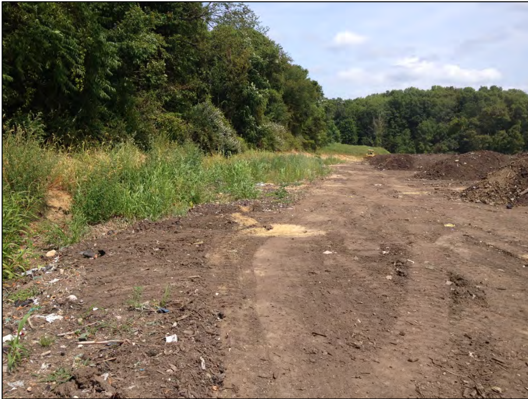
Photo 26: Proximity (~20-30') of drainage swale to active roadway and compost rows at the AgChoice stockyard.
