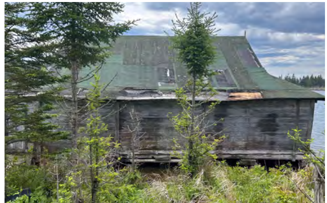
Figure 2-23. Roofing covering missing at north eave (source: Anderson Hallas, 2024).
