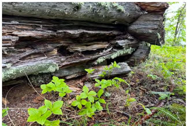
Figure 4-30. Logs in contact with soil (source: JVA, 2024).
