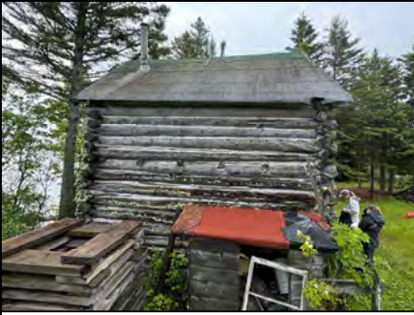
Figure 6. Distortion and roofing in poor condition at west façade (source: Anderson Hallas, 2024).
