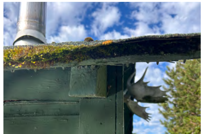
Figure 3-19. Bio-growth on sheathing at east eave (source: Anderson Hallas, 2024).
