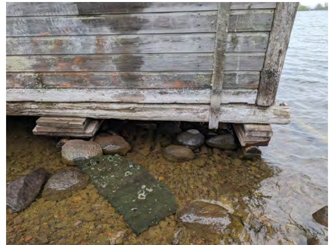
Figure 2-29. Tilting shims and loss of rock ballast (source: AMI, 2024).
