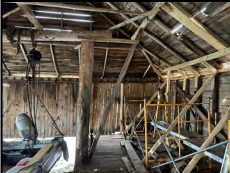
Figure 6. Broken rafters and shoring (source: JVA, 2024).
