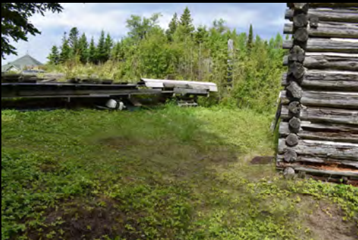
Figure 1. Low point along the south façade of Johns Log Cabin (source: Mundus Bishop, 2024).
