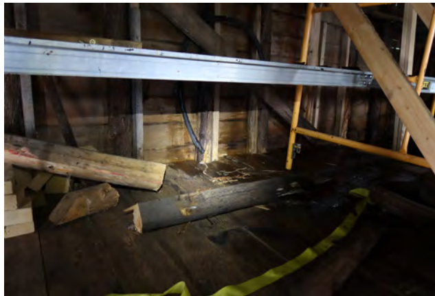
Figure 2-26. Water on interior floor decking, base of north wall (source: Anderson Hallas, 2024).
