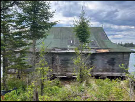
Figure 2. Roofing missing at north eave (source: Anderson Hallas, 2024).
