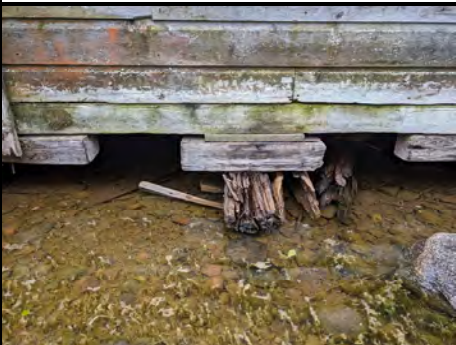
Figure 4. Crushed timber member (source: AMI, 2024).
