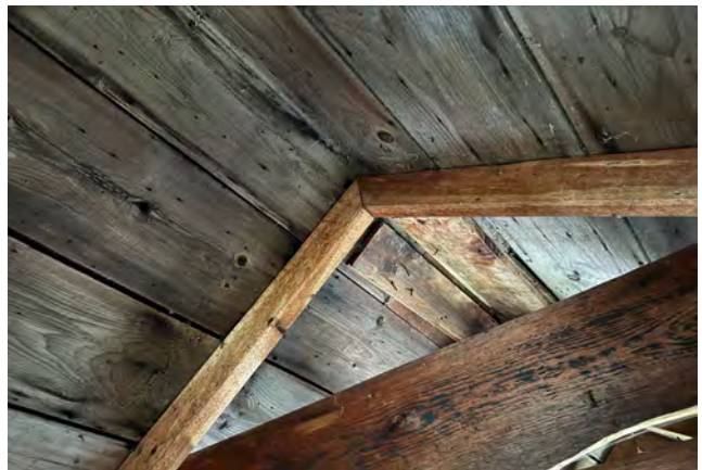
Figure 4-35. Roof rafters with a lack of ridge member (source: JVA, 2024).
