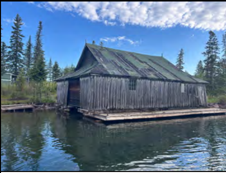
Figure 1. Missing and/or deteriorated roof coverings on south slope (source: Anderson Hallas, 2024).
