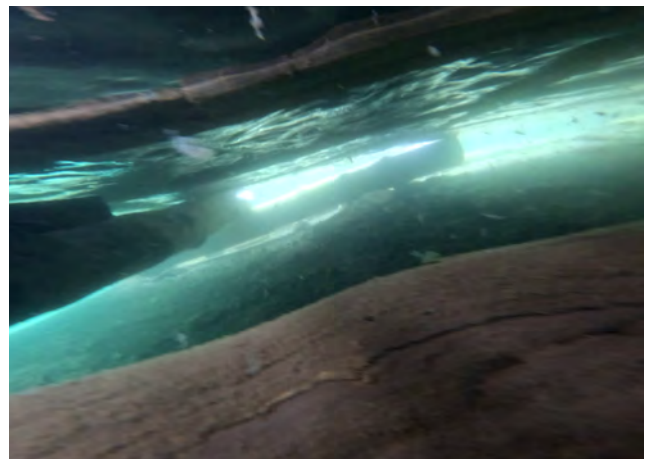
Figure 3-27. Loss of rock ballast (source: AMI, 2024).
