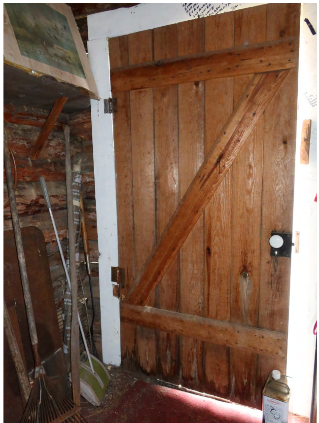
Figure 4-22. Exterior entry door, with window boarded with plywood (source: Anderson Hallas, 2024).
