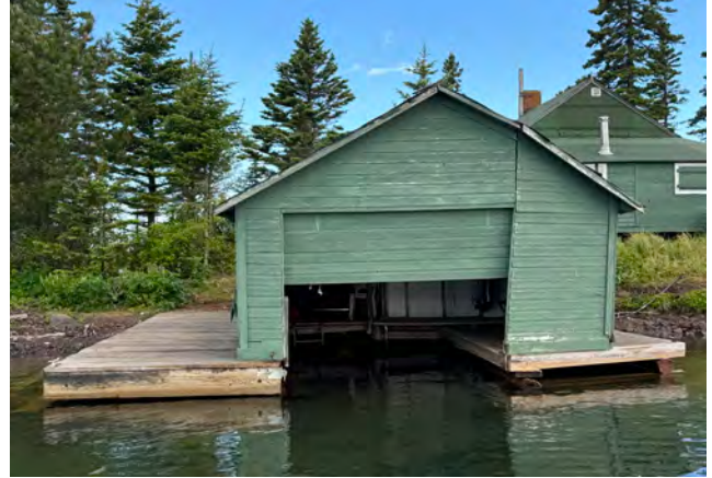
Figure 3-34. South wall elevation showing east wall leaning (source: JVA, 2024).
