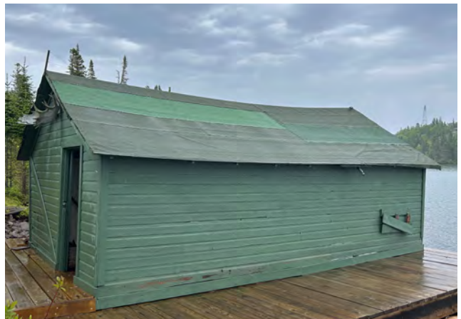
Figure 3-18. Wrinkled asphalt roll roofing, viewed from west (source: Anderson Hallas, 2024).
