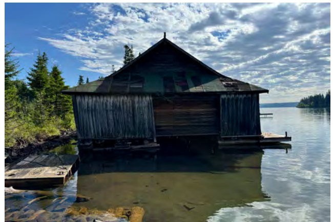
Figure 2-40. West wall elevation showing north wall leaning (source: JVA, 2024).
