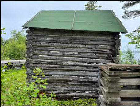
Figure 5. Distortion and roofing in poor condition at east façade (source: Anderson Hallas, 2024).
