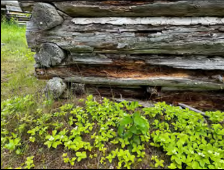
Figure 3. Lower logs in contact with soil, and no foundation (source: JVA, 2024).
