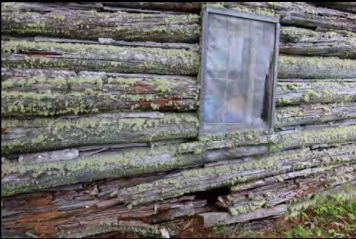
Figure 2. Deterioration at north façade (source: Anderson Hallas, 2024).
