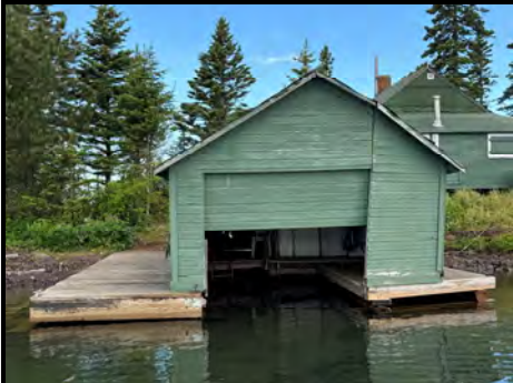
Figure 6. South wall elevation showing east wall leaning (source: JVA, 2024).
