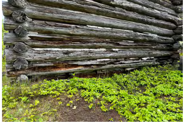
Figure 4-29. Lower logs in contact with soil, and no foundation (source: JVA, 2024).
