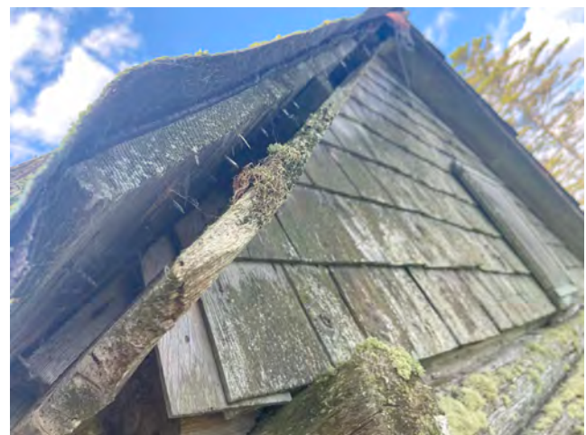
Figure 4-24. Soffit and missing barge board on north rake (source: Anderson Hallas, 2024).
