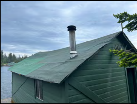
Figure 1. Wrinkled asphalt roll roofing, viewed from east (source: Anderson Hallas, 2024).
