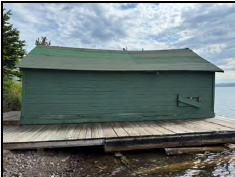
Figure 5. West elevation showing ridge sagging and wrinkled roof covering (source: JVA, 2024).
