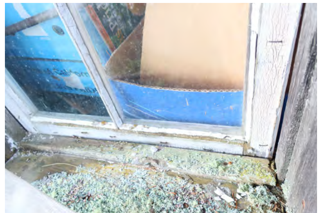
Figure 4-20. Deteriorated paint and putty at first-floor north window (source: Anderson Hallas, 2024).
