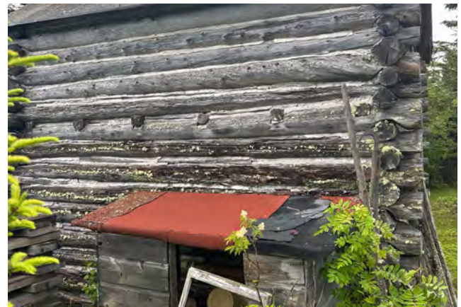
Figure 4-16. Bio-growth at west façade (source: Anderson Hallas, 2024).
