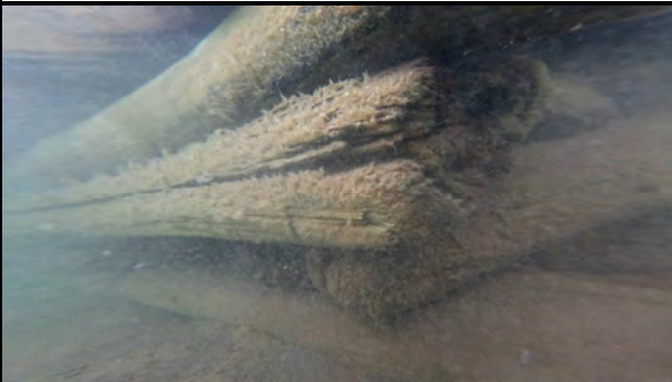
Figure 3. Lower crib member deterioration (source: AMI, 2024).
