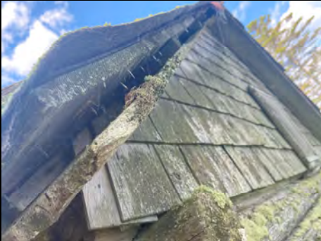
Figure 4. Soffit and missing barge board unsupported and roof covering excessively overhanging sheathing on the north rake (source: Anderson Hallas, 2024).
