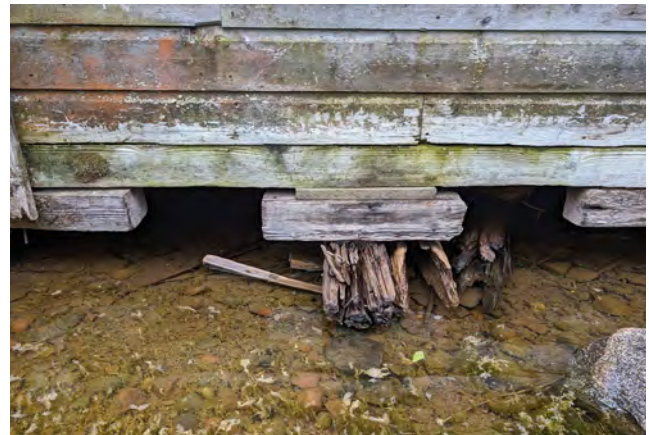
Figure 2-28. Crushed timber member (source: AMI, 2024).
