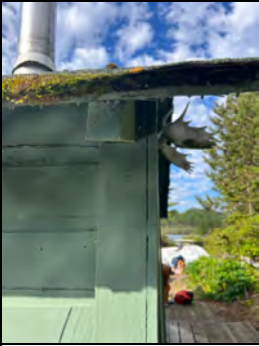
Figure 2. Bio-growth and deterioration at east eave (source: Anderson Hallas, 2024).
