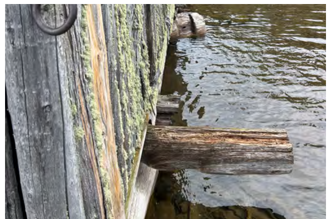
Figure 2-15. Lichen and bio-growth on west exterior wall (source: Anderson Hallas, 2024).
