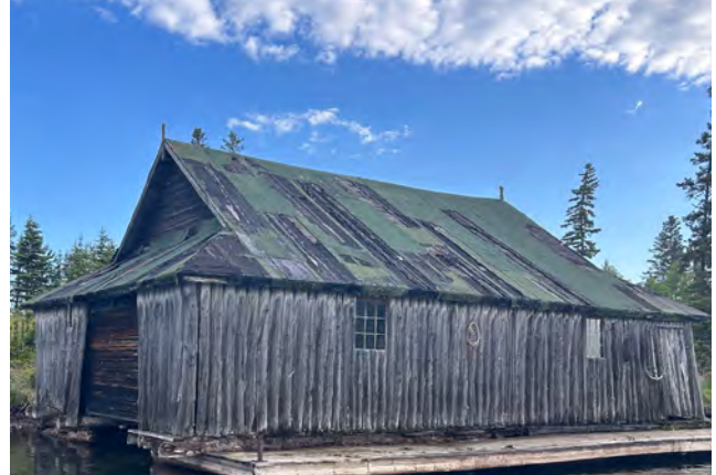
Figure 2-22. Missing roof coverings on south slope (source: Anderson Hallas, 2024).
