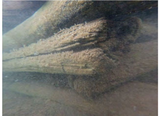
Figure 3-26. Lower crib member deterioration (source: AMI, 2024).
