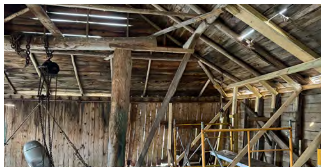
Figure 2-32. Broken rafters and shoring (source: JVA, 2024).
