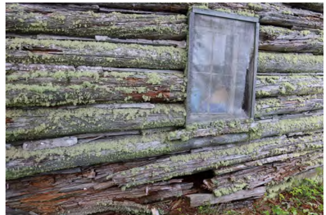
Figure 4-17. Deterioration at north façade (source: Anderson Hallas, 2024).
