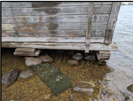
Figure 5. Tilting shims and loss of rock ballast (source: AMI, 2024).
