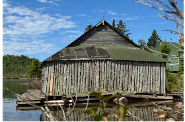
Figure 2-39. East wall elevation showing significant structural movement (source: JVA, 2024).
