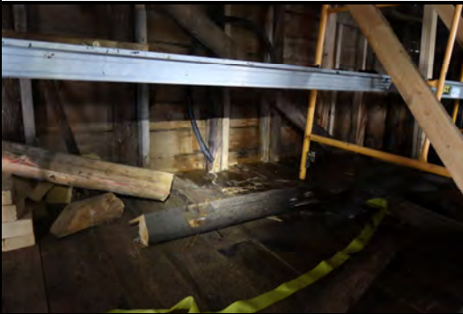
Figure 3. Water intrusion at base of north wall (source: Anderson Hallas, 2024).
