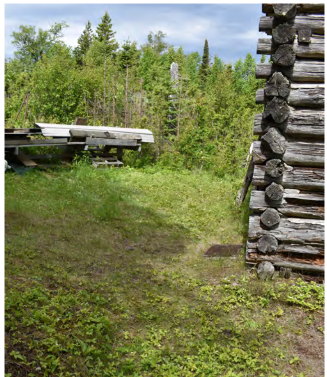
Figure 4-5. Low point along the south façade of Johns Log Cabin (source: Mundus Bishop, 2024).
