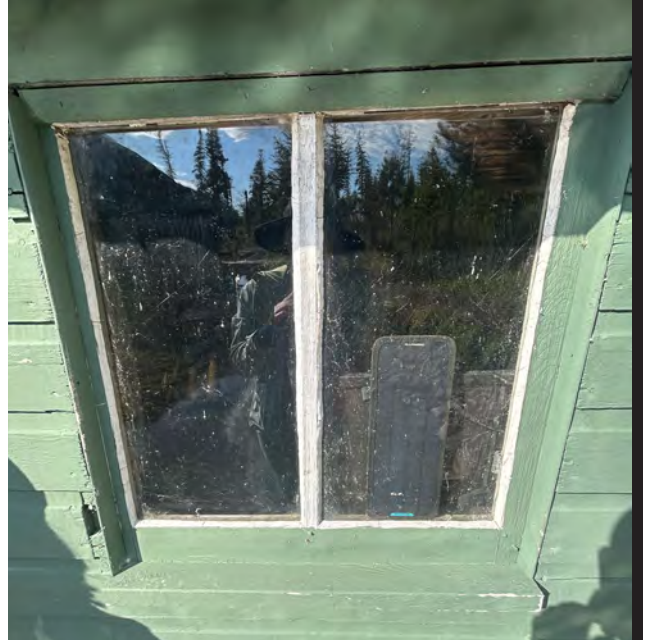
Figure 3-13. Missing trim around window (source: Anderson Hallas, 2024).
