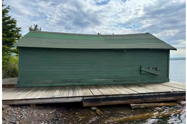
Figure 3-31. West elevation showing ridge sagging (source: JVA, 2024).
