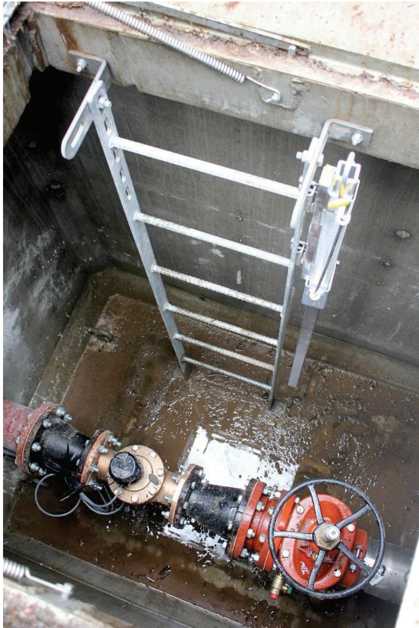
Photograph 13: Looking down into meter and valve vault for Well #3 (fire well) (NPS/2019).
