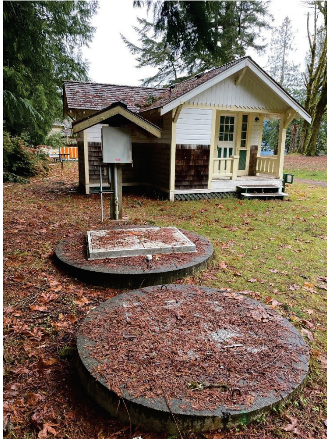
Photograph 11: Lift Station No.2 and valve vault near Dardanella Cabin at Rosemary Inn Campus, looking north (NPS/2024).
