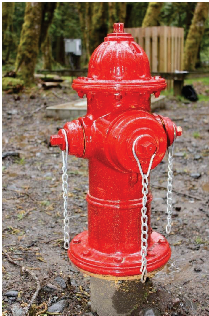
Photograph 14: Typical fire hydrant along water system, Well #3 seen in background, looking northwest. (NPS/2019).
