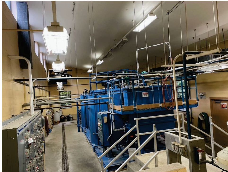
Photograph 4: Interior of Treatment Room of Barnes Point Wastewater Treatment Plant, looking west (NPS/2024).
