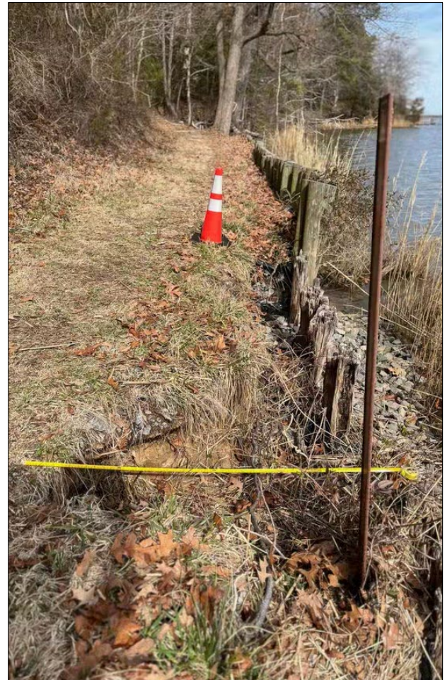
Figure 3. Trail Erosion Behind the Timber Wall (erosion is up to 3 feet wide)
