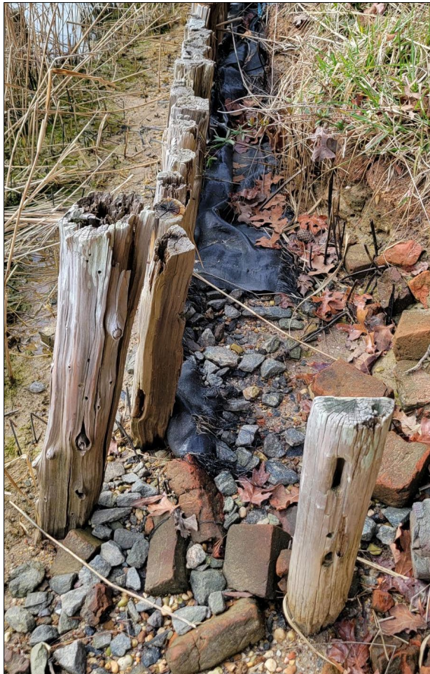
Figure 2. Timber Wall Scour Revealing Geotextile Fabric and Fill Material
