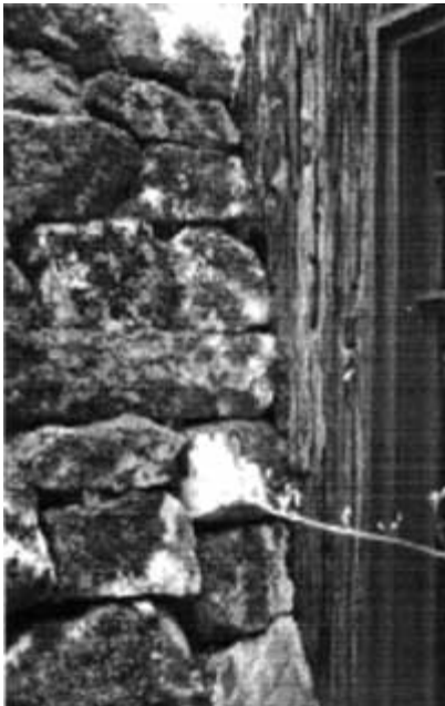
Moss growth at southeast corner.
