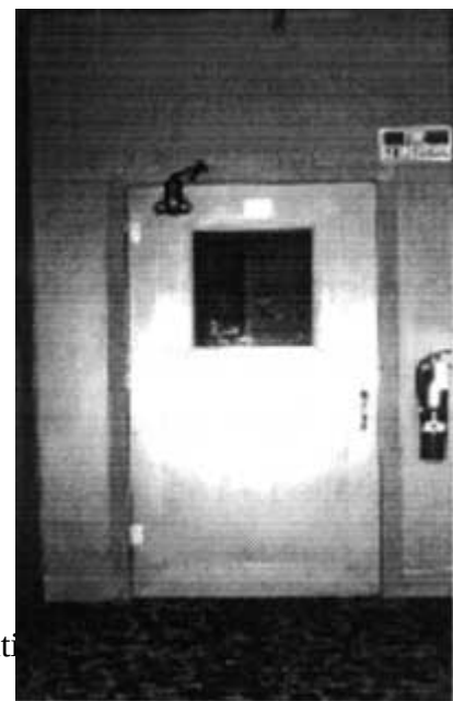
Typical Chateau fire door.
