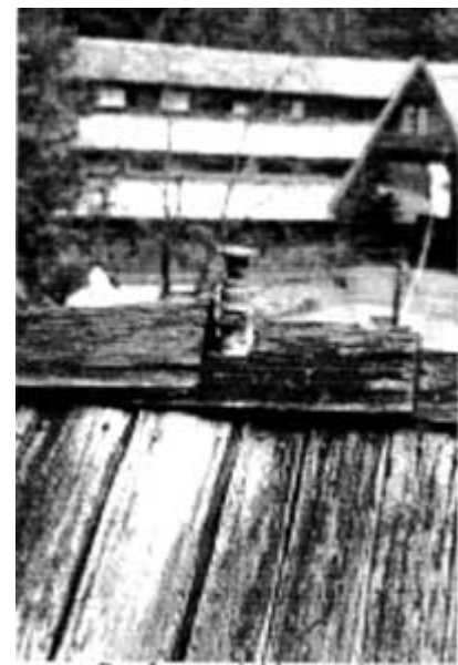
Small dormer, west side. Note the damage.
