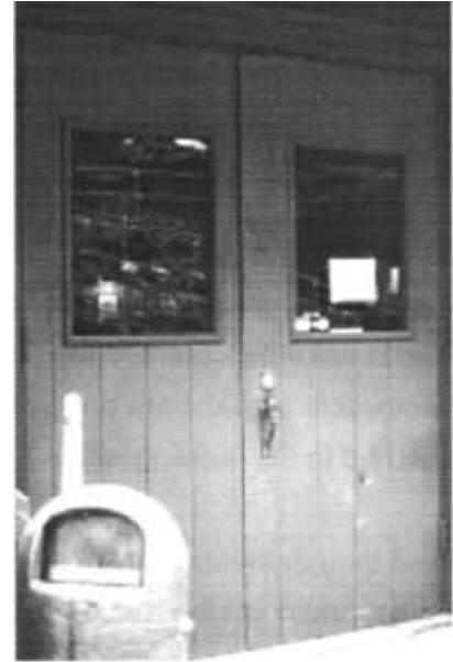
Lobby entrance doors. Note the bow.
