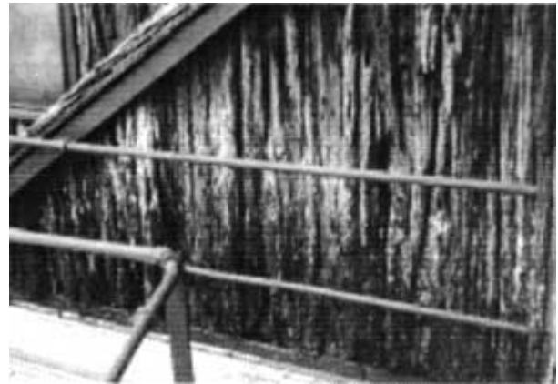
Growth at west stair enclosure.
