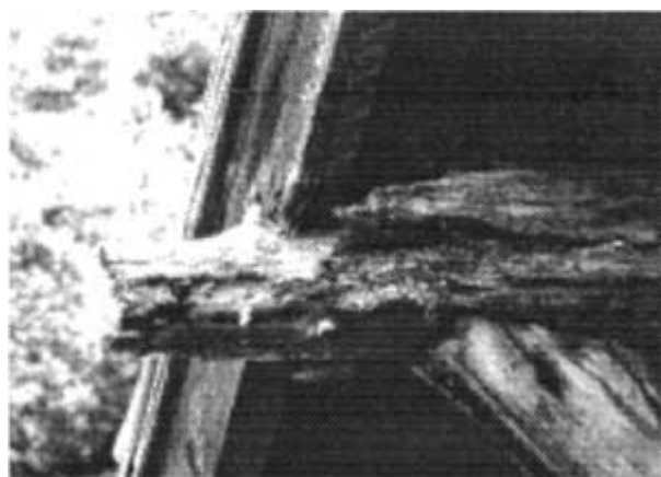
Typical decay of gable bracket end.
