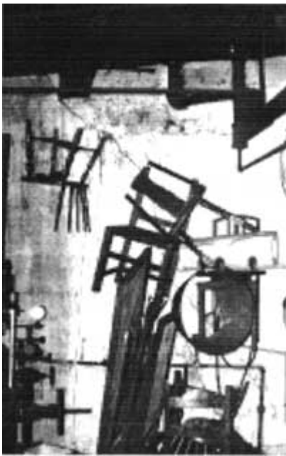
Crack in the boiler room, north wall.
