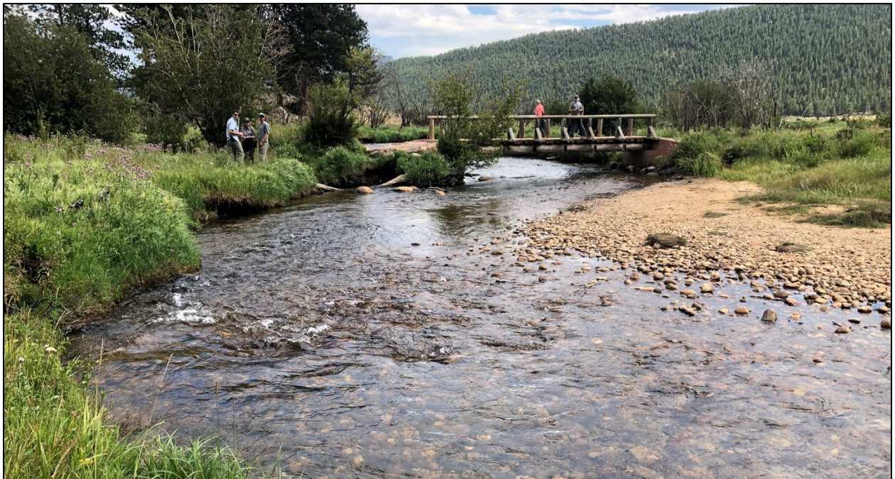
Figure 4. Downstream view of the Big Thompson River. The active channel width (i.e., bankfull width) is much wider than the bridge opening. The cut bank at left of the bridge will probably migrate downstream reclaiming the active channel width. This will surround the north bridge abutment and likely necessitate anti-scour measures. NPS, 2019.
