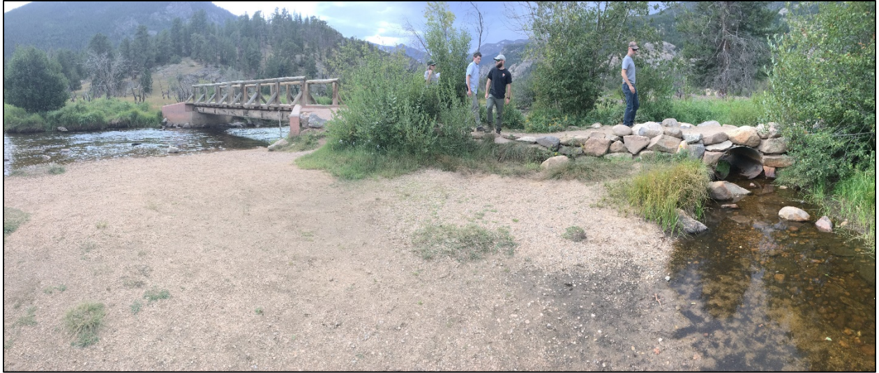
Figure 3. Upstream view of the Cub Lake trail, the bridge over the mainstem Big Thompson River, the prism of fill, and the culvert on the side-channel. The fill acts as a barrier to in-channel and overland flow at higher discharges. Note the large boulders that could serve as point protection riprap. NPS, 2019.
