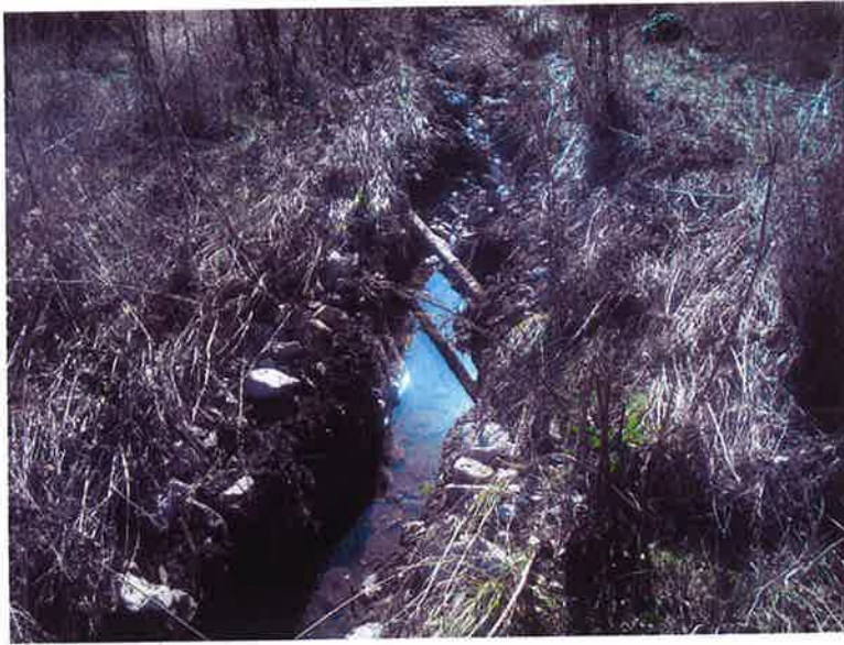
Figure 4. Reach of Chalone Creek where it has undergone incision, exposing a previously buried utility line
