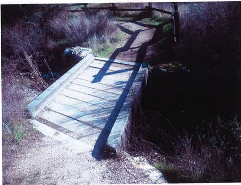
Figure 5. View of the small footbridge that could be the cause of the incision. Note the encroachment of the abutment on the far bank.
