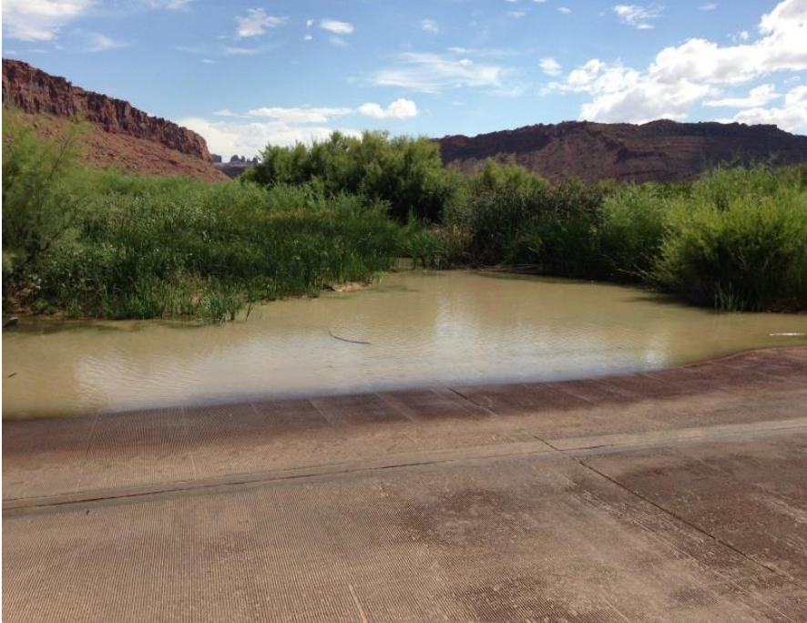
Figure 5. Salt Valley Wash looking downstream from the road crossing. Note that the culvert outlet is completely submerged due to downstream aggradation and vegetation establishment. NPS – 2016.
