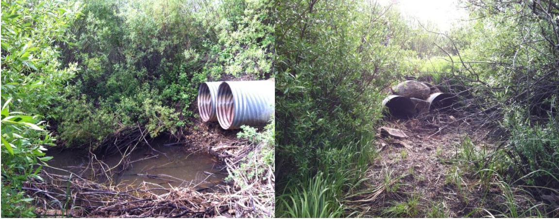
Figure 2 – culvert crossing that passes through the road fill. The left image is the downstream side (note the plunge pool. On the right image, the upstream side, note the accumulation of sediment.
