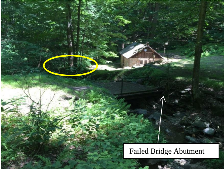
Figure 4 - The historic Ike Smith Pump House (1936) that serves as water distribution for Park facilities. The yellow ellipse marks several riparian trees that will probably be lost relatively soon without treatment. Note the vehicle access bridge that has failed on the right bank side. (NPS-2017)
