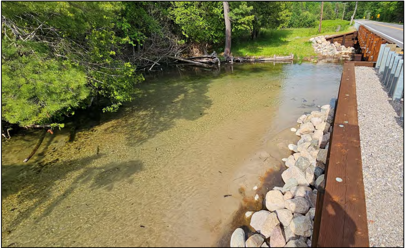
Photo B-43. View immediately downstream of Crossing 3, June 12, 2025. SWCA noted a significant increase in fine sand in this area.
