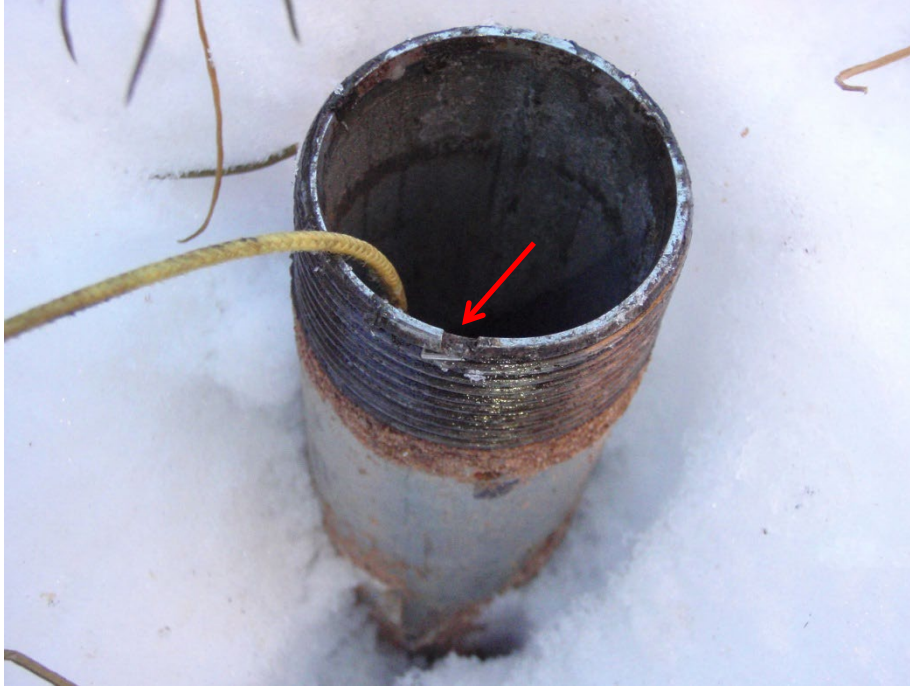
Figure 5. The measuring notch on the well casing
