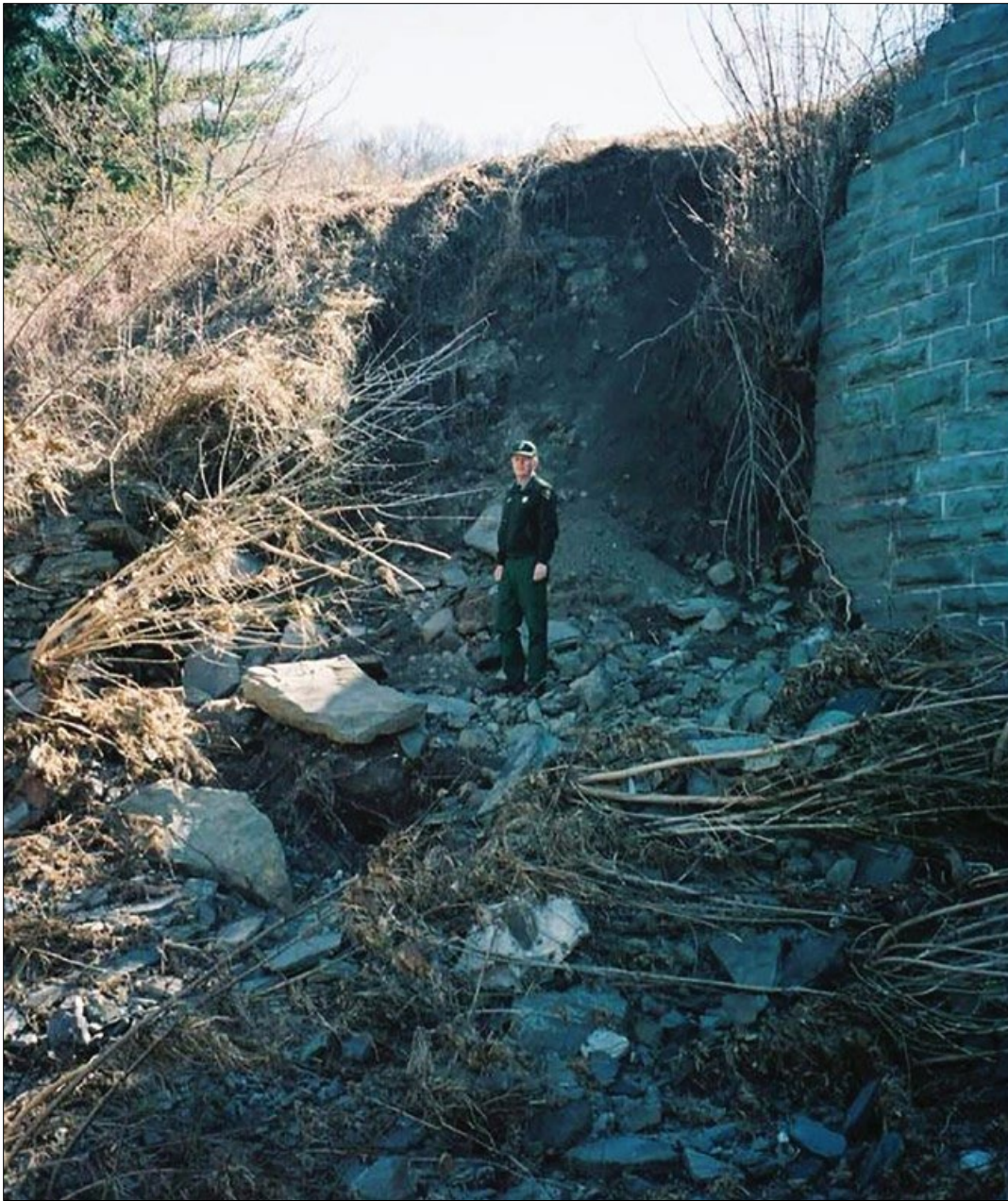
Figure 13. Flood damage sustained to Roebling's Delaware Aqueduct in 2005. Hurricane Ivan in September 2004 and excessive rainfall in April 2005 produced near-record flooding and partially collapsed the aqueduct/bridge's stone wing wall extending upstream (north) from the New York side abutment. NPS employee for scale. Figure 1.81 from Killion et al. (2023).
