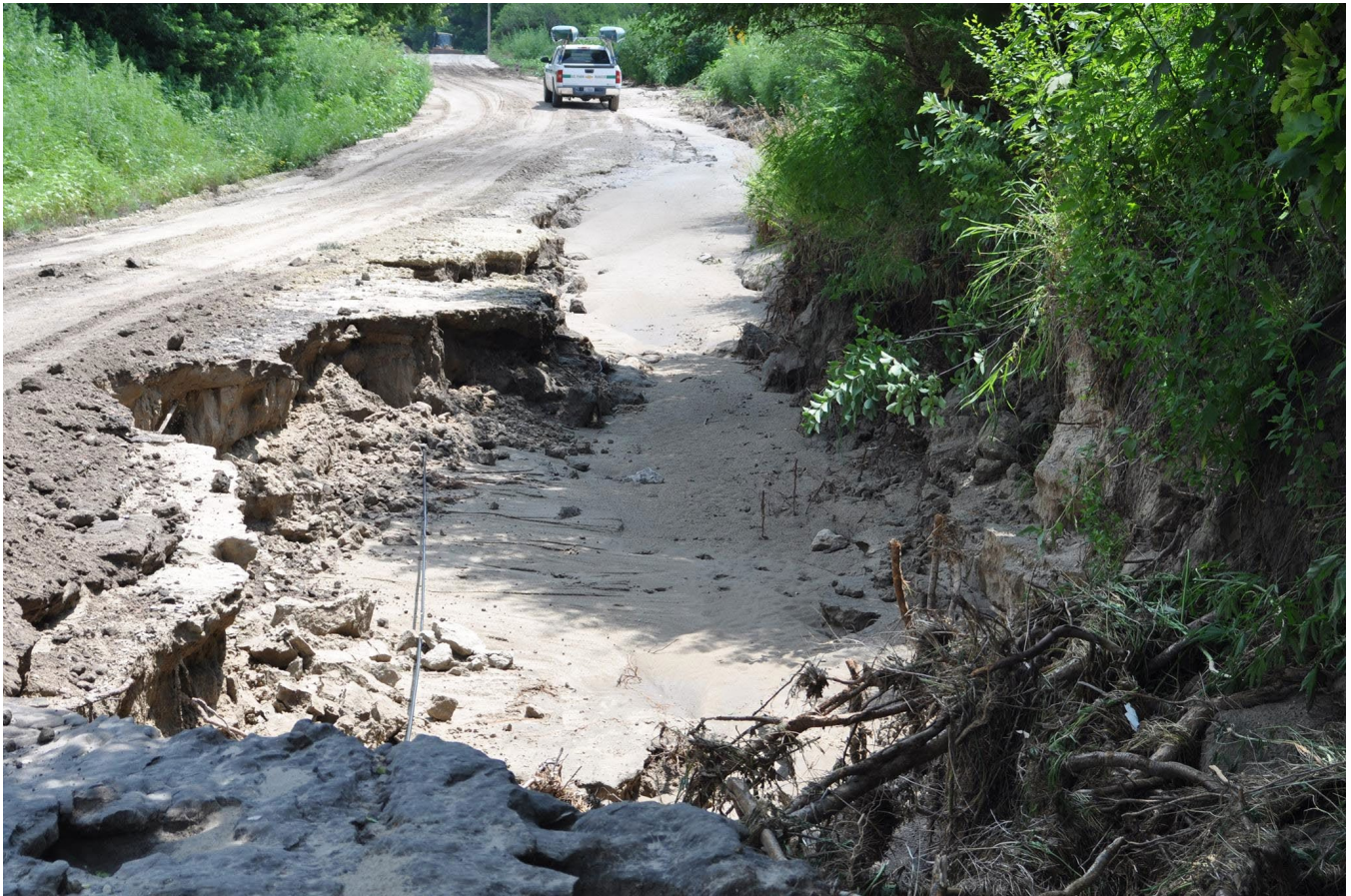
Figure 13. Photograph of a partial washout between Sharp's and Stan's landings in July 2013. Enhanced runoff undercut and washed away a portion of the roadway, leaving behind unconsolidated rocky and vegetative debris. NPS photograph.
