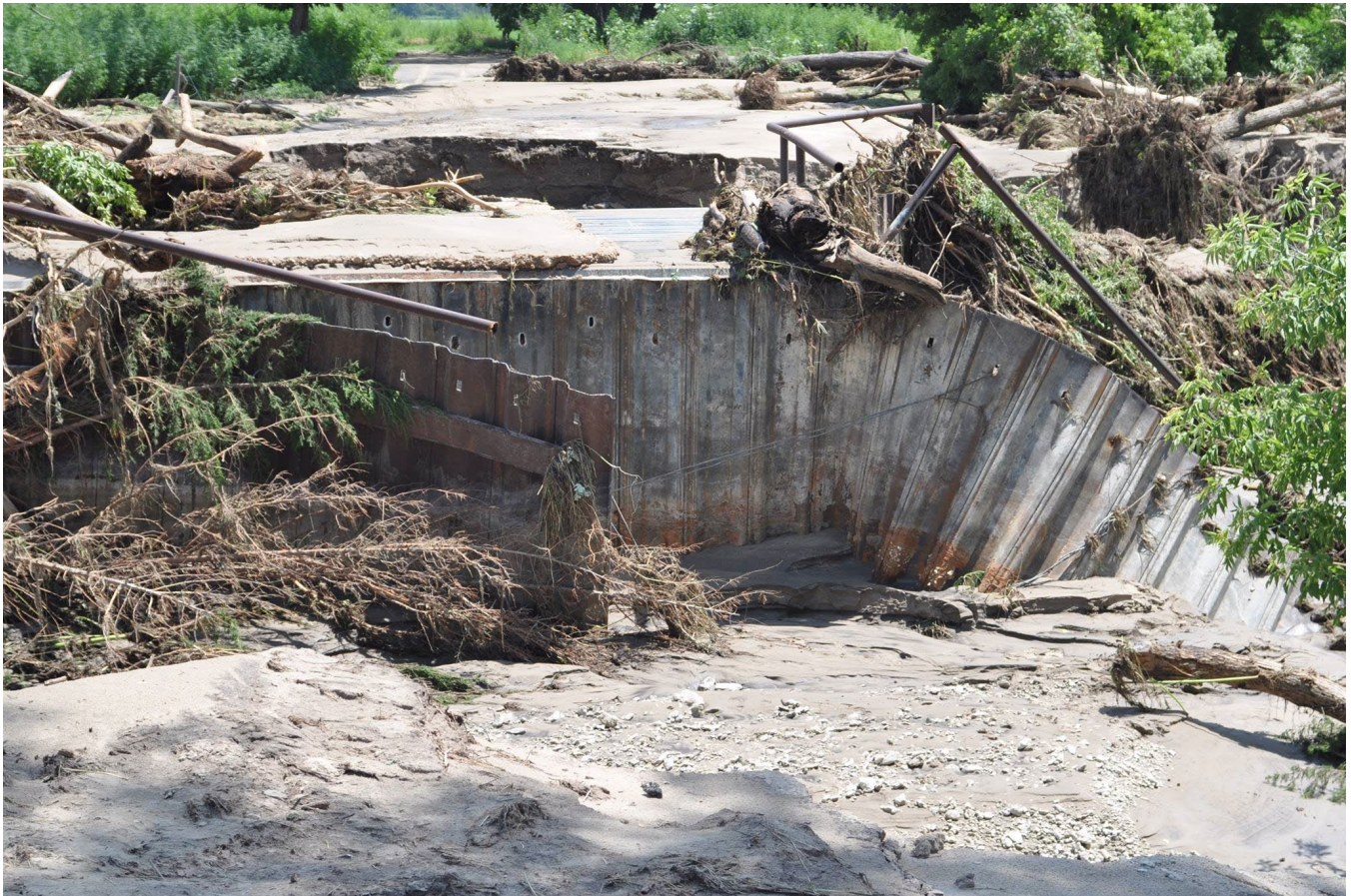
Figure 14. Photograph of a bridge washout following July 2013 flooding. The bridge is located immediately east of Sunny Brook Camp along River Road. An unnamed tributary damaged the bridge and deposited mud, silt, rock, and vegetative debris along the roadway surface. NPS photograph.
