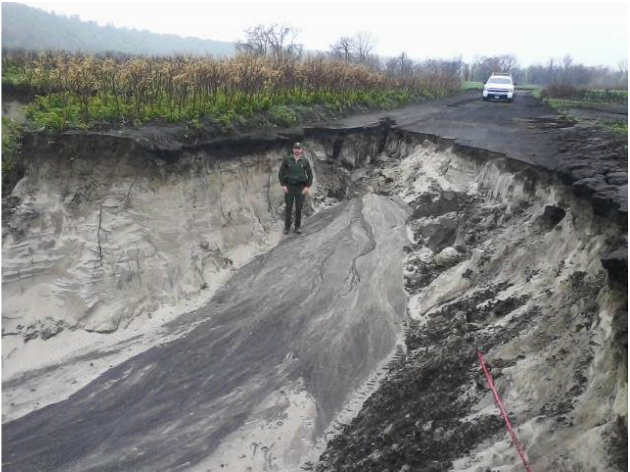
Figure 12. Photograph of a washed-out segment of River Road in June 2013. The washout occurred approximately 1.6 km (1 mi) east of the Norden Bridge and exposes the lower terrace alluvium of the Niobrara River. Enhanced runoff and flooding undercut and washed out a sizeable section of the roadway, making it impassable. NPS employee for scale. NPS photograph.
