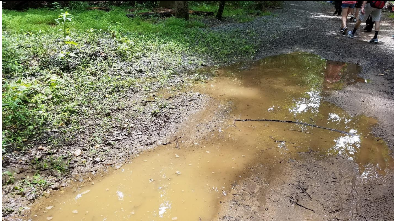
Figure 23: Standing water in depression in the gravel road to Theatre in the Woods.
