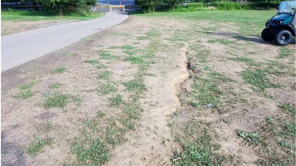
Figure 19: Sediment erosion on Gill's Hill.
