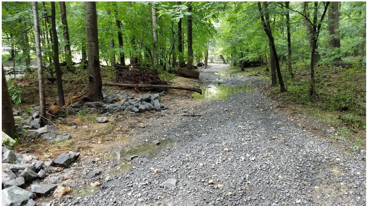
Figure 24: Gravel road to Theatre in the Woods following July 8 th flood.
