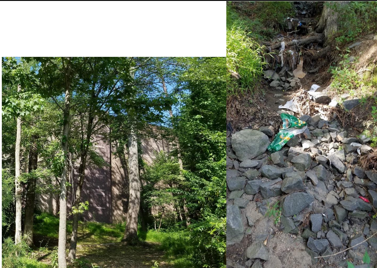
Figure 18: (Left) Area adjacent to Lot 4 previously clear cut to access noise barrier wall for repair and location of one of two culverts draining into the park. Heavy runoff makes reestablishment of vegetation difficult. (Right) Ditch which carries runoff from Dulles Toll Road towards West Lot during storm events.
