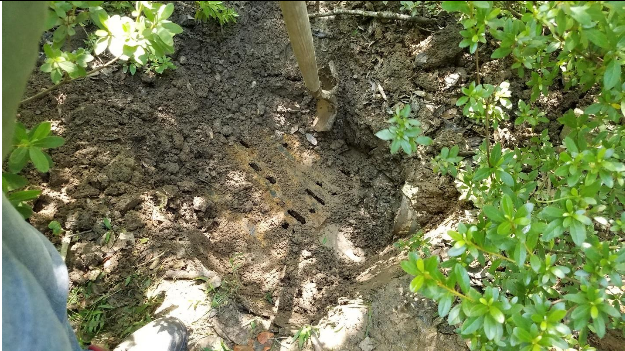
Figure 22: Worker excavates a storm drain adjacent to the Filene Center which had been buried by sediment eroding from uphill.
