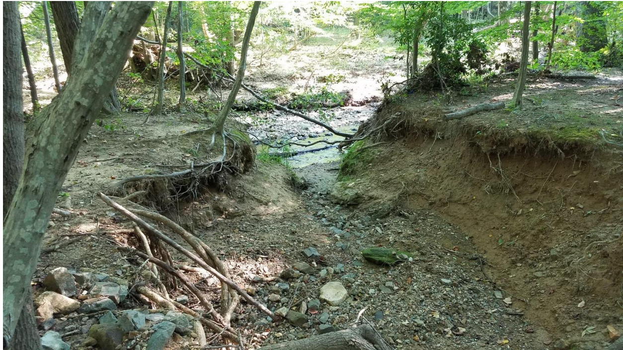
Figure 27: Outlet of eroded ditch in figure 26 into Wolf Trap Creek.
