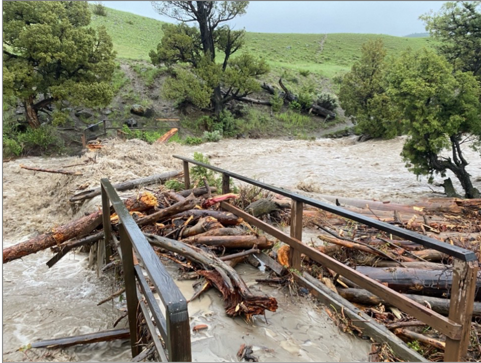
Figure 14. Washed-out bridge at Rescue Creek, Yellowstone National Park. NPS / CHRIS FLESCH
