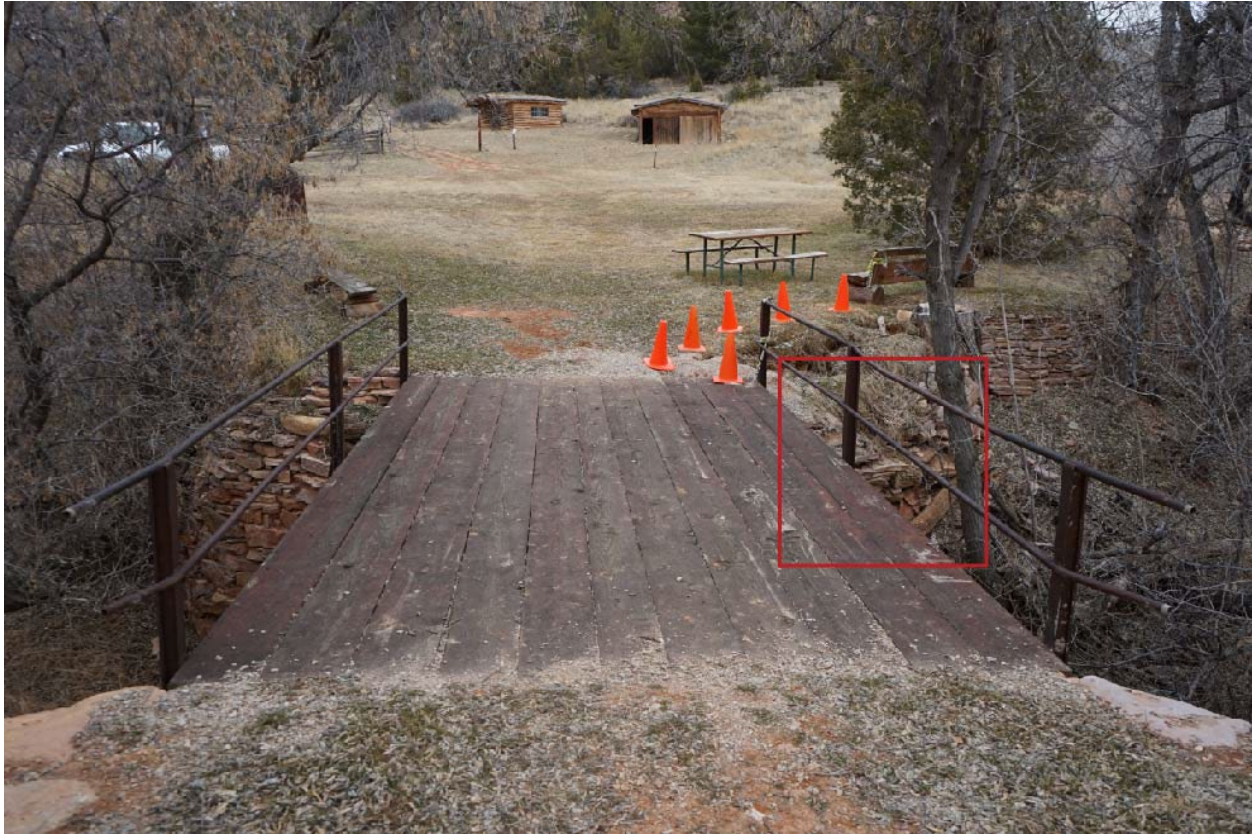
Figure 3 - East side of bridge where the dry stack and logs have almost completely failed.
