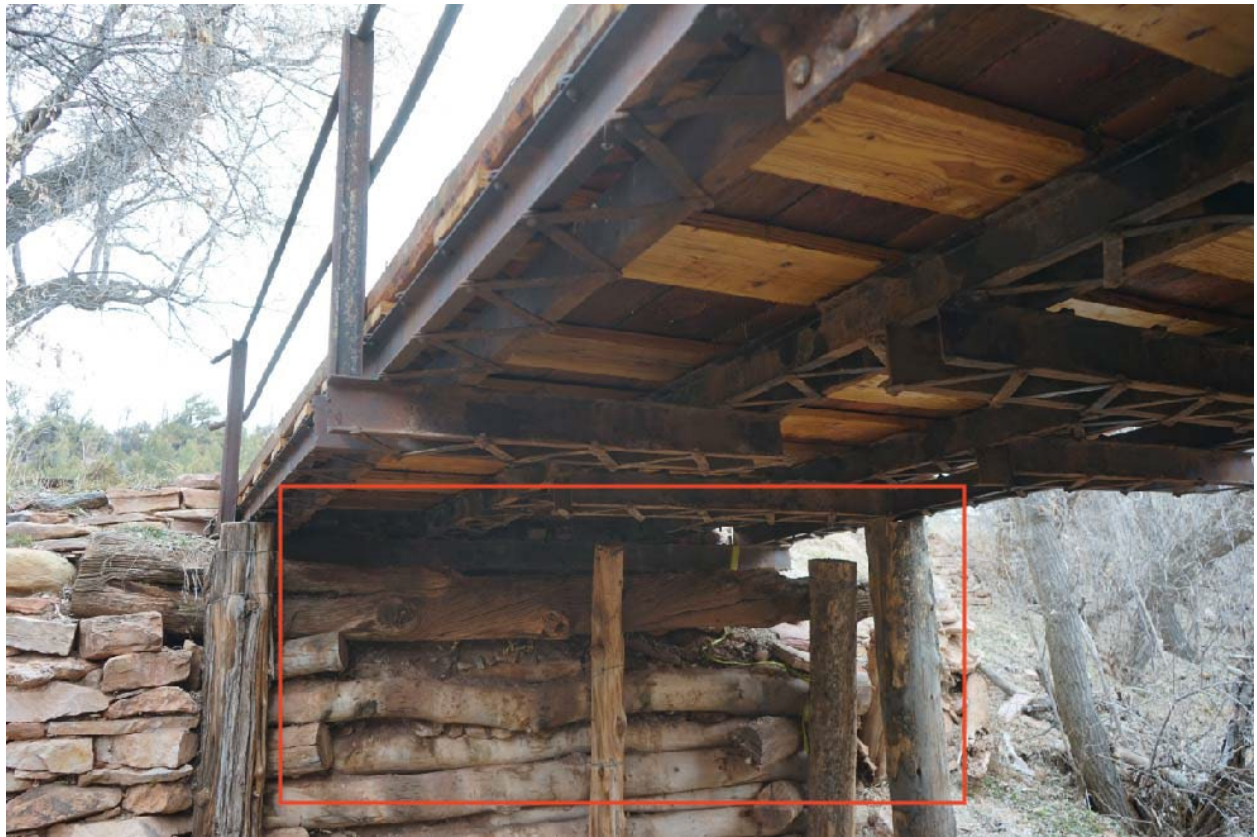
Figure 1 - North side of bridge showing failing logs and wash out behind the logs that is compromising bridge stability.
