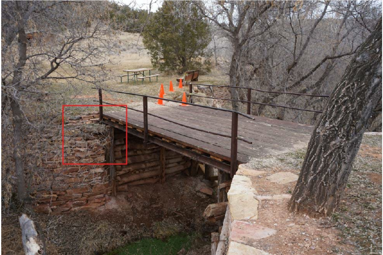
Figure 2 - Dry stack starting to fail on west side of bridge. Locations will be restacked before damage gets worse.
