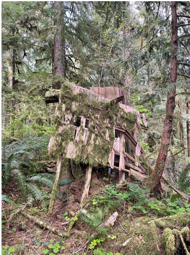
Photograph 18: Collapsed gable roof of stump privy, northeast of house, looking east (NPS/Matsov, 2025).
