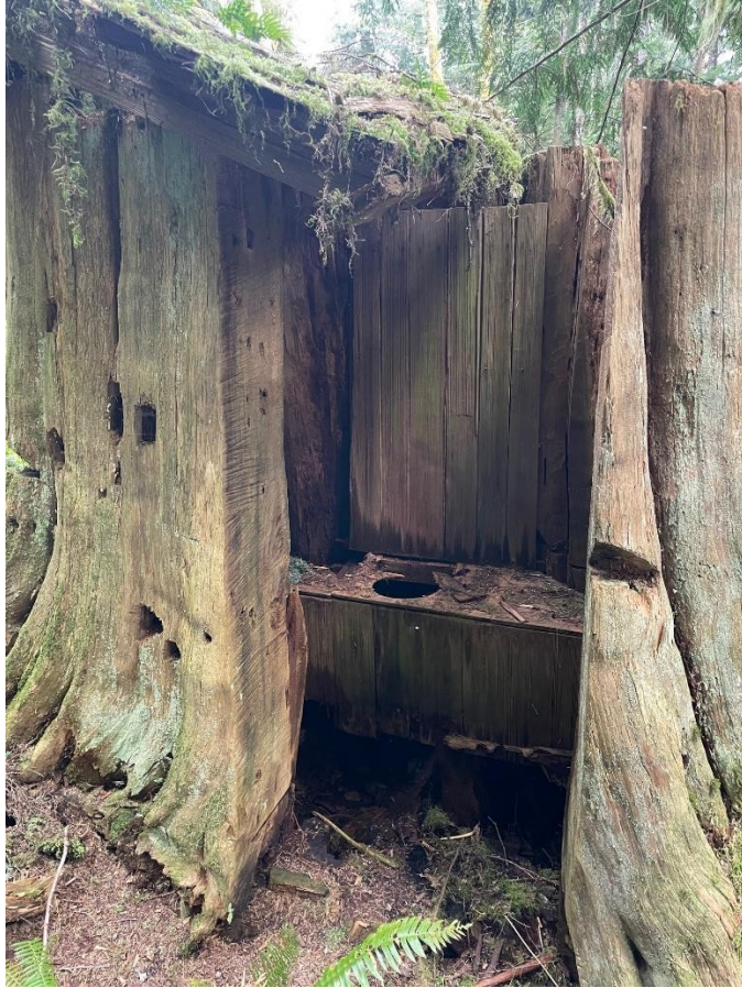
Photograph 19: Cut entry into privy, showing seat and collapsed gable roof (NPS/Matsov, 2025).
