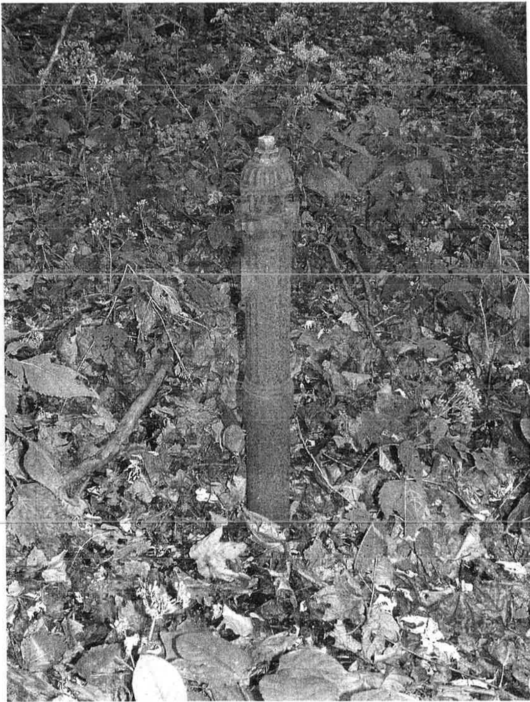
Figure 44: Fire hydrant at Hamlet IHTIA, 2003
