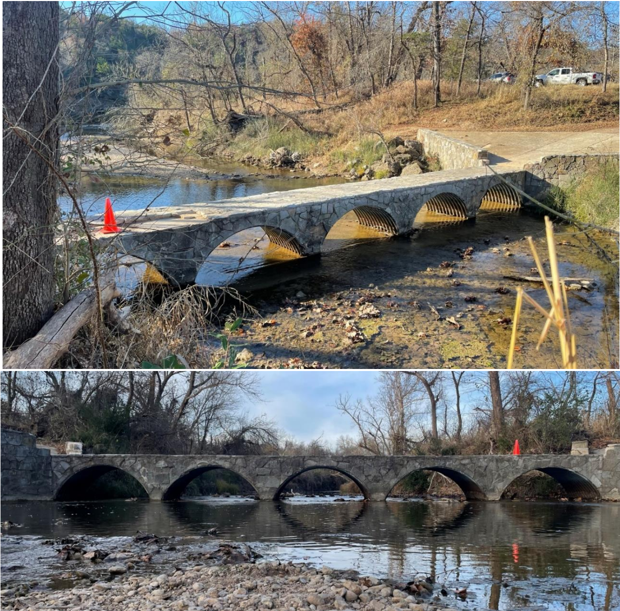
Figure 4. Photos looking downstream (top) and upstream (bottom) at the Job Corps Bridge. High flows frequently overtop the bridge and pose a threat to visitors.
