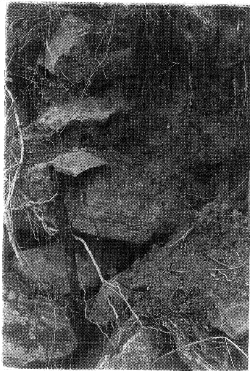
Fig. 14. Material of slopes has filled interstices of riprap.
