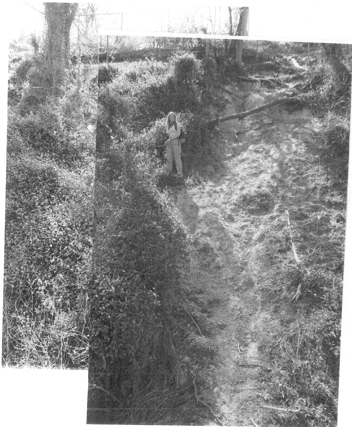
Fig. 8. Slope D. Immediately east of Redoubt #10. Heavily vegetated area on left, unstable footpath on right.
