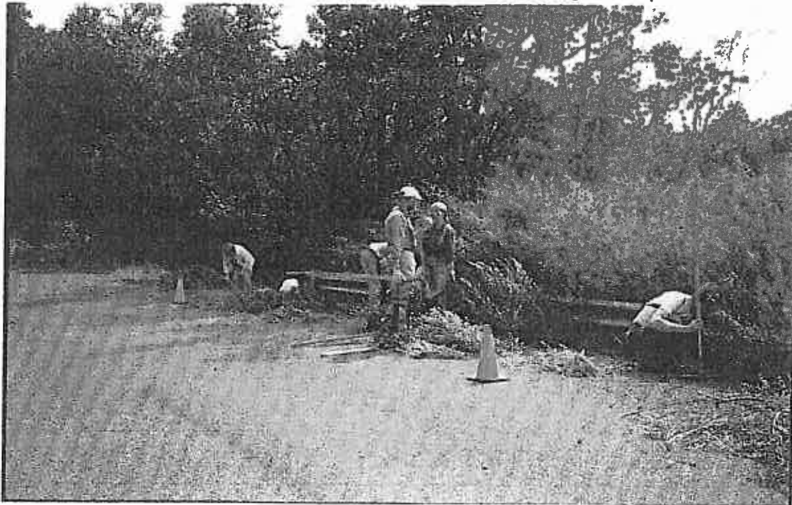
Figure 8. Broom removal at the scrub-dominated landslide area along Bolinas-Fairfax Road in 1992. Photo by M. Alvarez.
