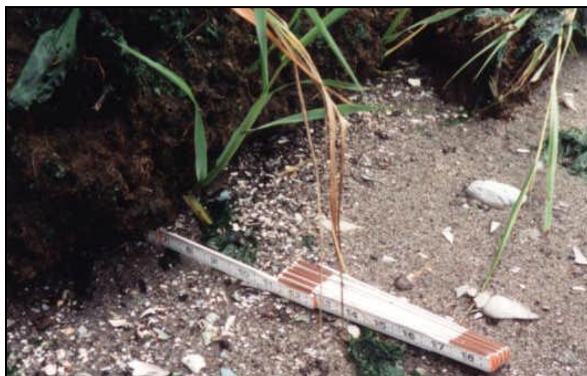
Fig. 8. Extent of undercutting of low marsh embankment greater than 6 inches (15 cm) as indicated on carpenter's ruler.
