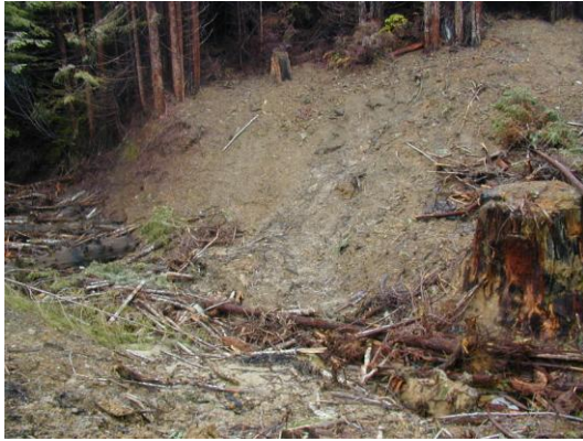
Photo 23: Post-excitation, early winter view of RX E3, after first set of heavy rains. View shows the fillsite failure along the left bank of the excavation.
