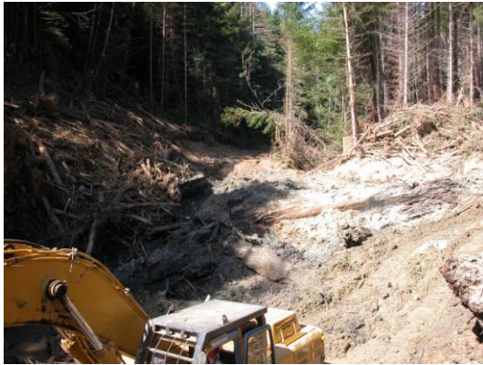
Figure 16a. Uncovering large ‘jackpot’ of woody debris in lower portion of B540
