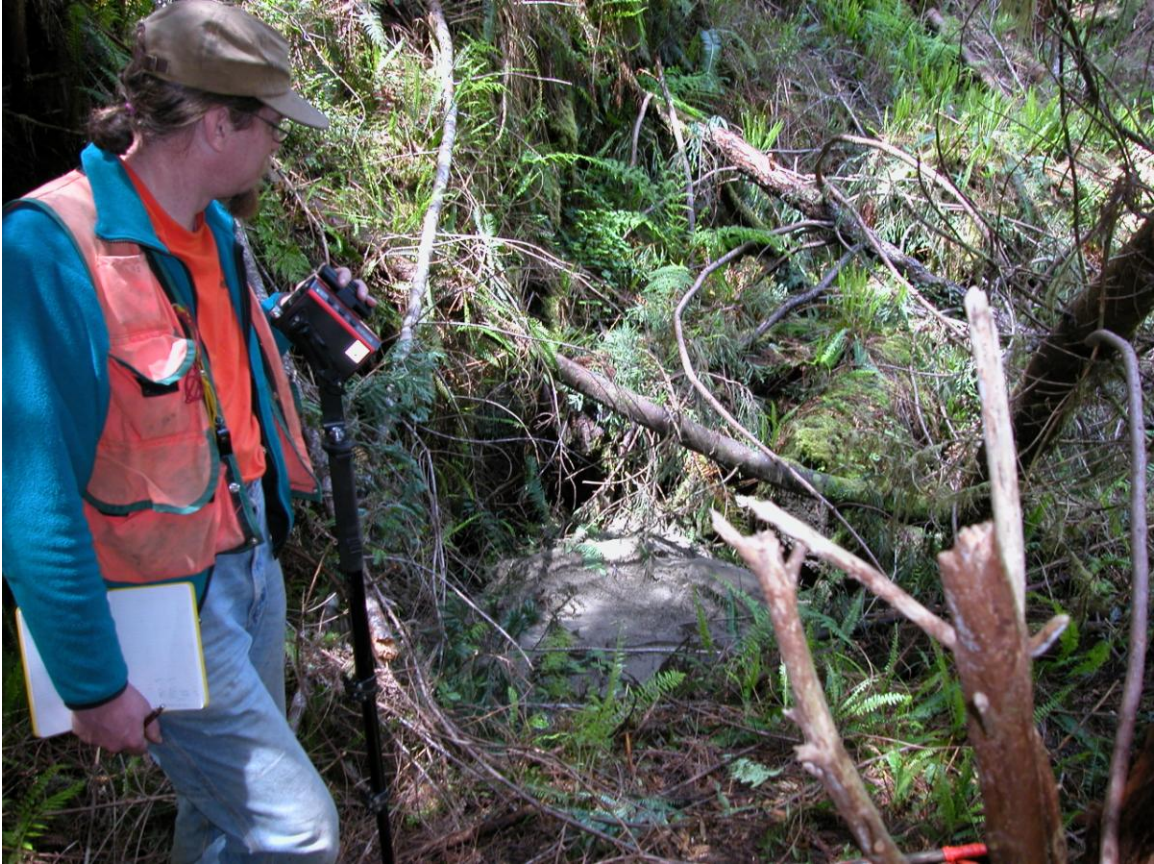
Figure 9. Sediment deposit in a hole at Upper Y derived from internal decay of crossing fill (field book for scale). Deposition is located approximately 3 feet above active flow at time of photo.
