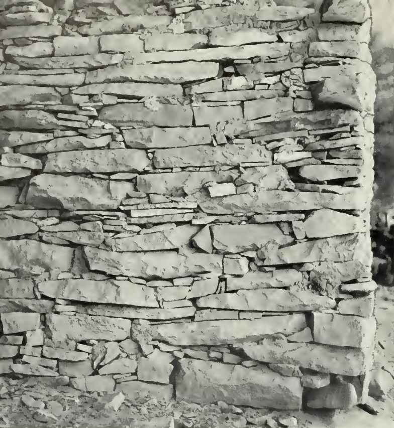
Figure 17—Wall of scabbled stone in "chipped edge" style. Many spalls but little mortar. Site 1446.
