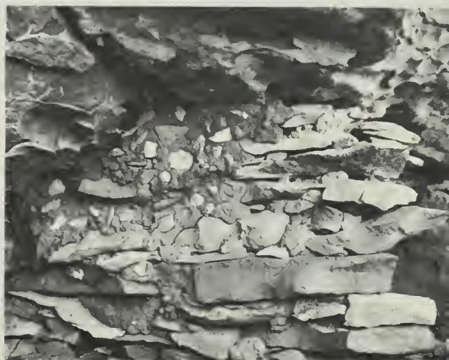
Figure 15—Wall of rough, unshaped rock and spalled adobe. Site 1504.
