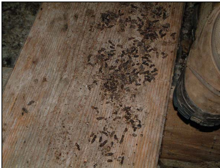
Figure 8. Small amounts of bat guano found on boards in Knox Tindle Farmhouse.
