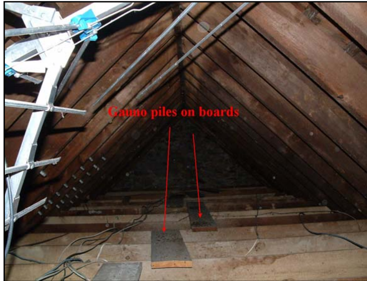
Figure 7. Small guano piles found on boards in the Knox Tindle Farmhouse.
