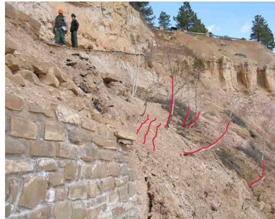
Figure 4b. The landslide annotated to show the tension cracks, scarps and “pistol butted” aspen trees on the slope highlighted in red.
