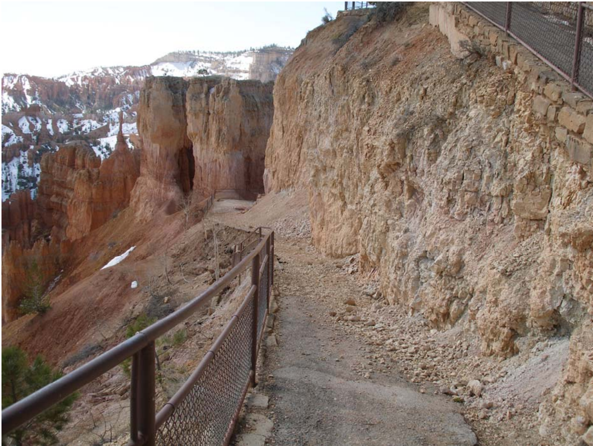
Figure 2. The rockcut and rockfall hazards at the top of the Navajo Loop Trail.
