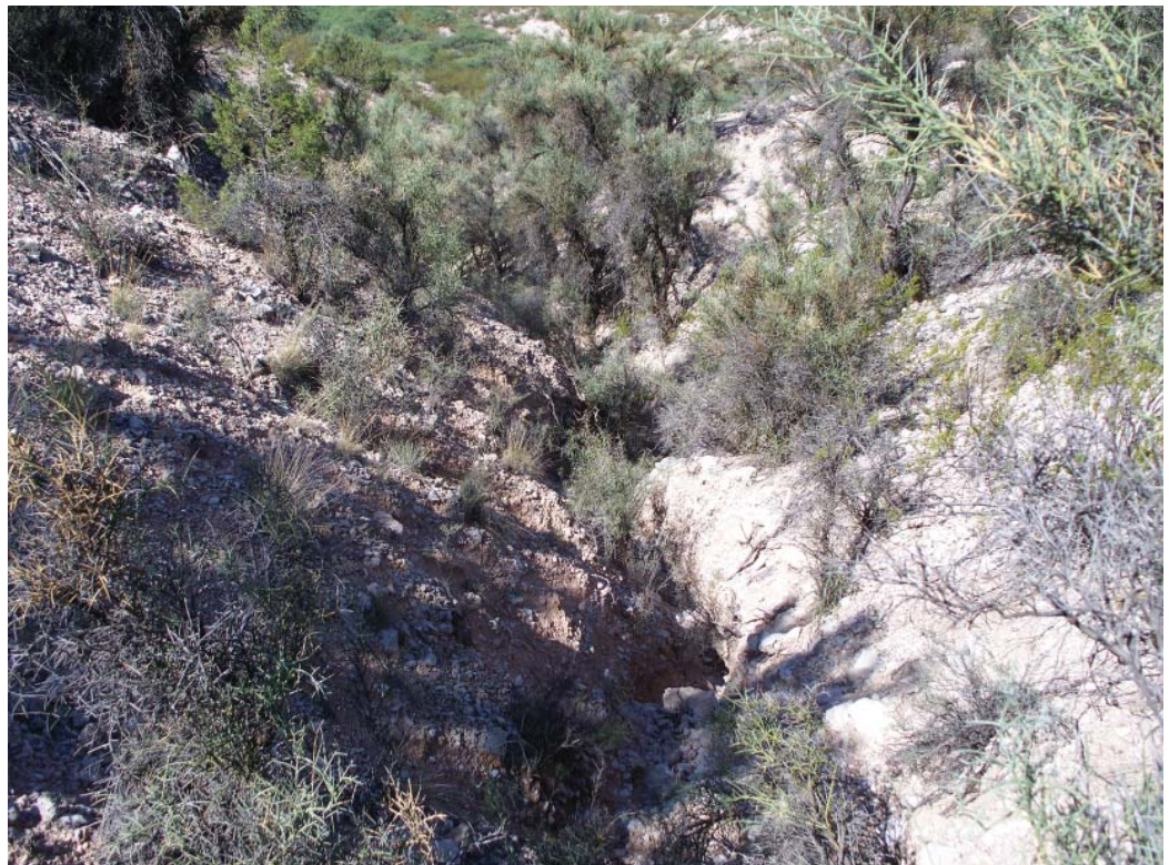
Figure 3.3.3. Gully in the northwestern-drainages area, showing an unstable sideslope above the actual cut.
