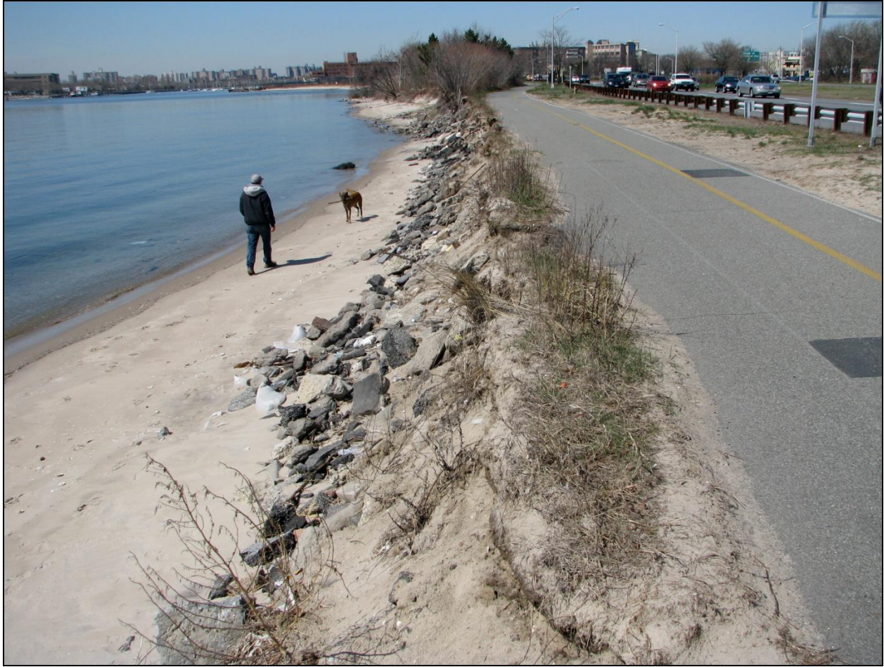
Figure 25. Riprap exposed at eroding sector, central Plumb Beach, March 31, 2009
