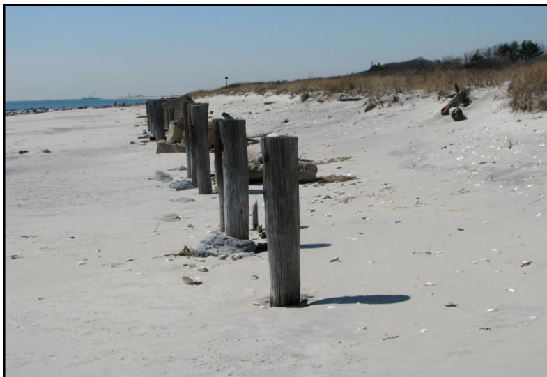
Figure 20. Portions of the wooden bulkhead and riprap wall exposed at base of foredune in Ft. Tilden. March 31, 2009.
