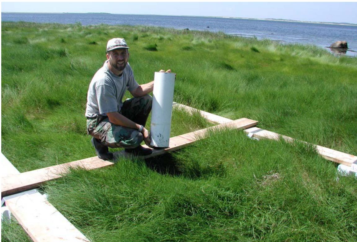
Figure 3.19. PVC collar (Barn Island, CT USA).
